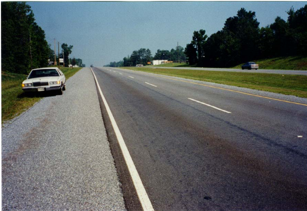
Figure 6. Tallapoosa Project - Granite Section Showing Moderate Flushing in Travel Lane (Left) and Slight Flushing in Passing Lane (Right)
