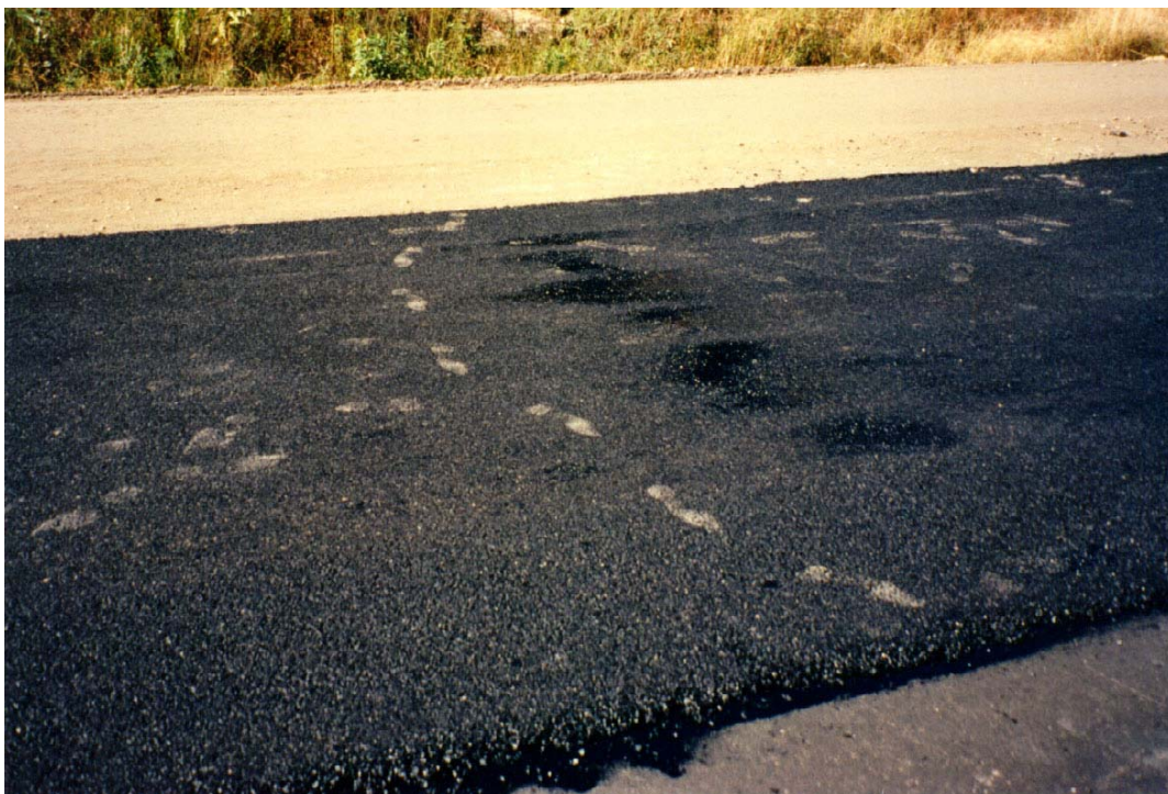
Figure 4. Tack Coat Puddles Where the Machine Stopped
