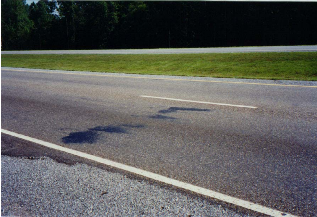
Figure 5. Tallapoosa Project - Flushing Due to Spray Bar Leakage
