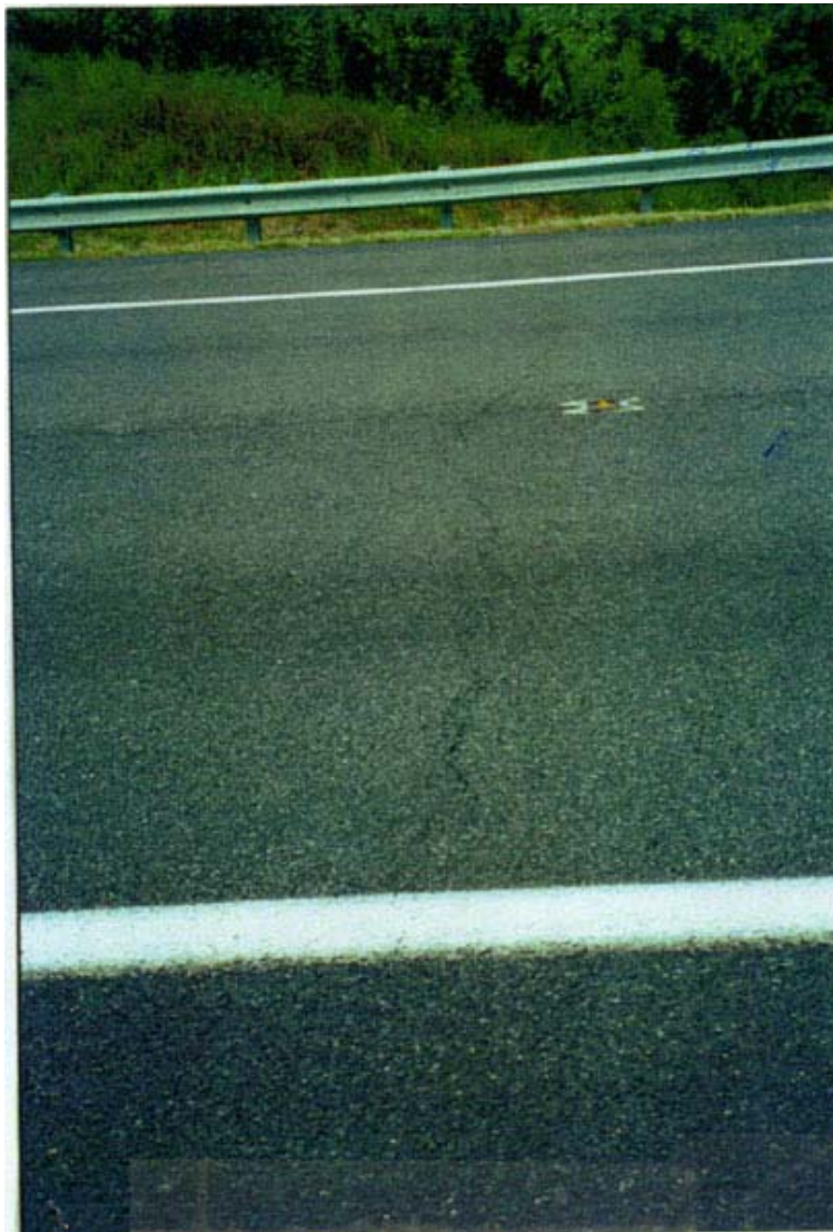
Figure 20. Typical Transverse Crack in SMA Mixture
