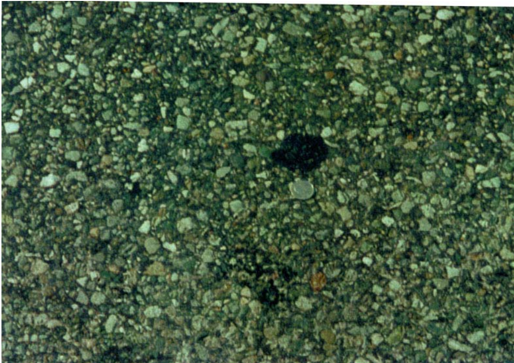
Figure 18. Small Blemish Caused by Build Up of Mortar on Screed
