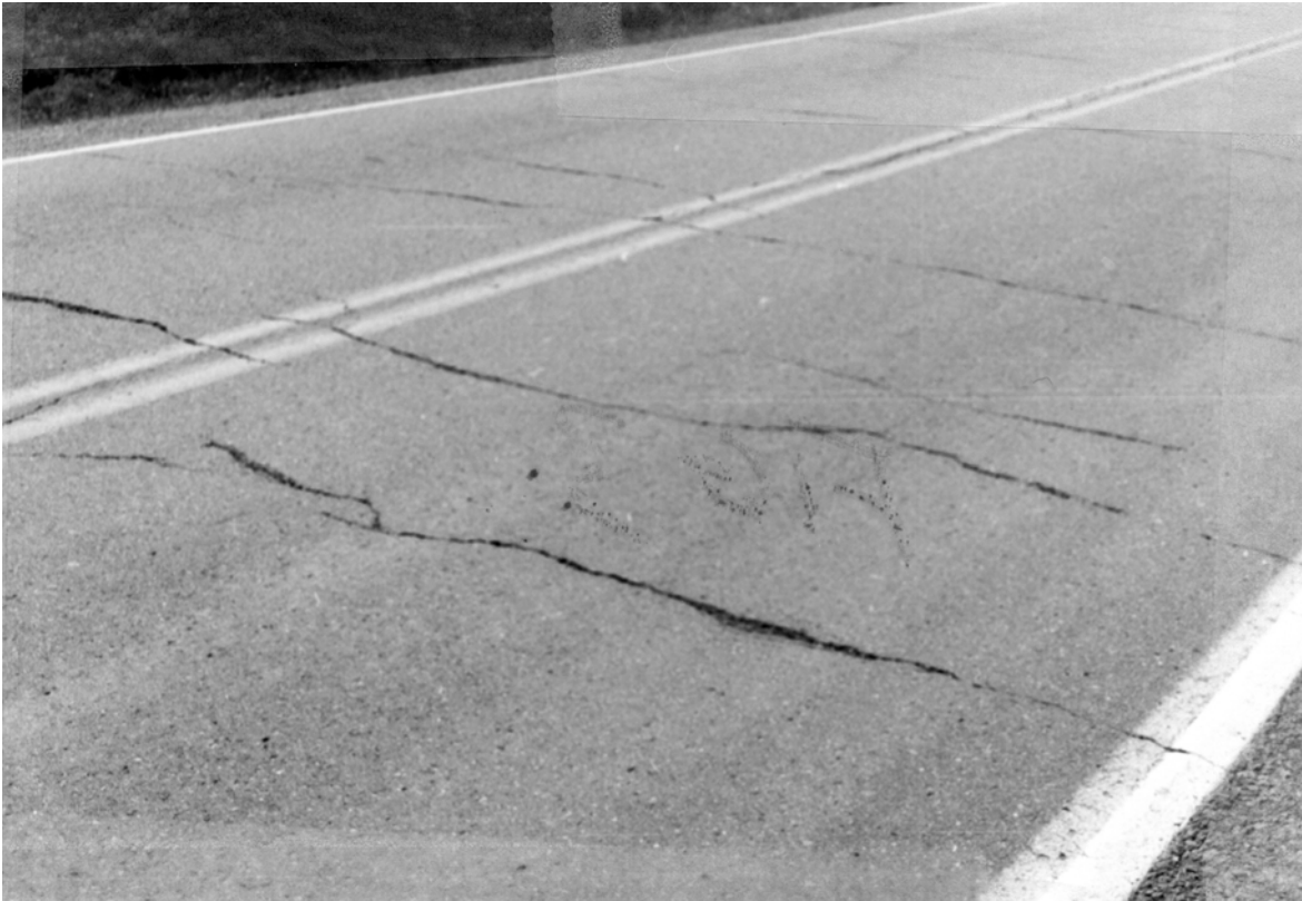
Figure 4. Asphalt T-5 in Both Lanes Showing Well-Defined Full and Half-Width Transverse Cracks
