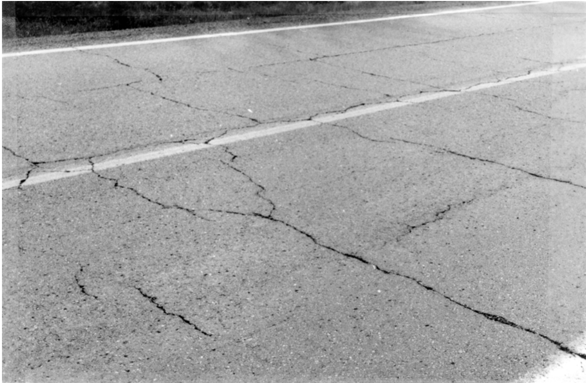
Figure 2. Asphalt T-1 in Both Lanes Showing Transverse Cracking
