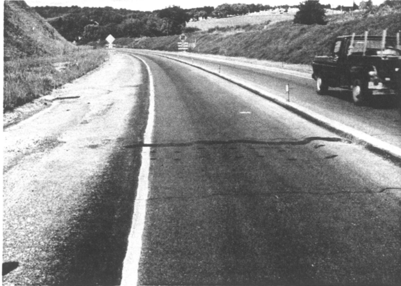
Figure 3. Rutting on I-70 Washington County (1986)
