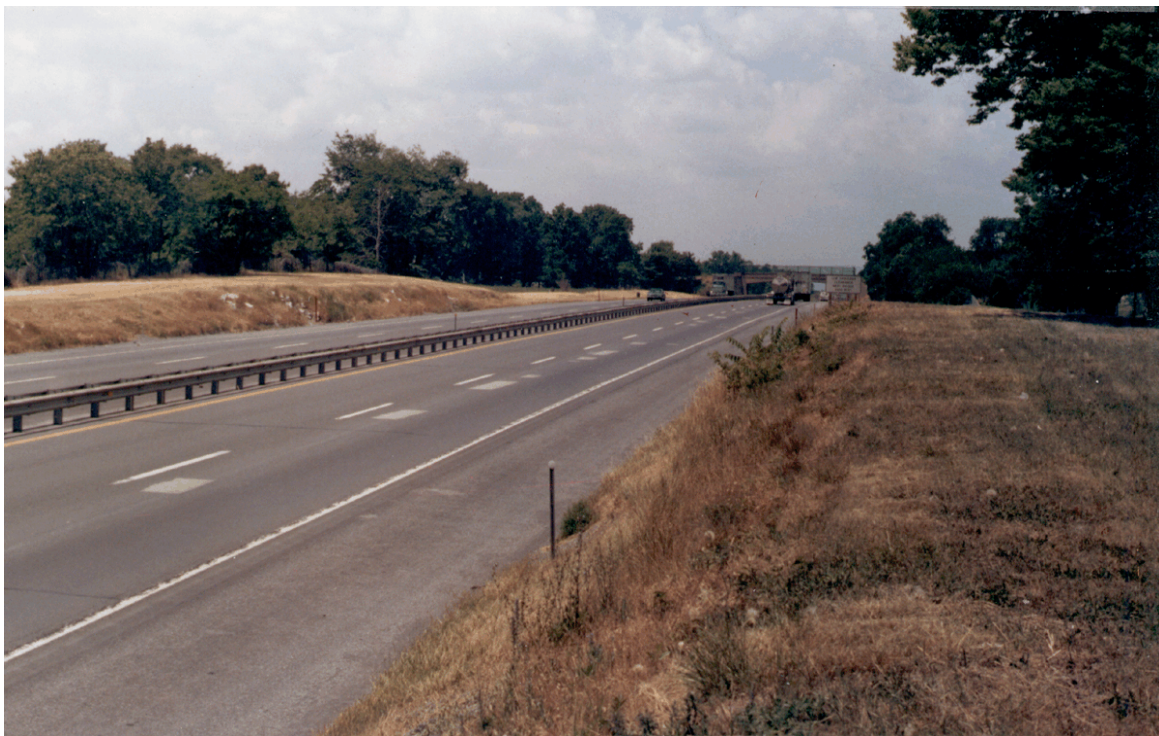
Figure 7. East-West Turnpike (General View Showing a Series of Patched potholes on Inside Wheel Track of Slow Lane)
