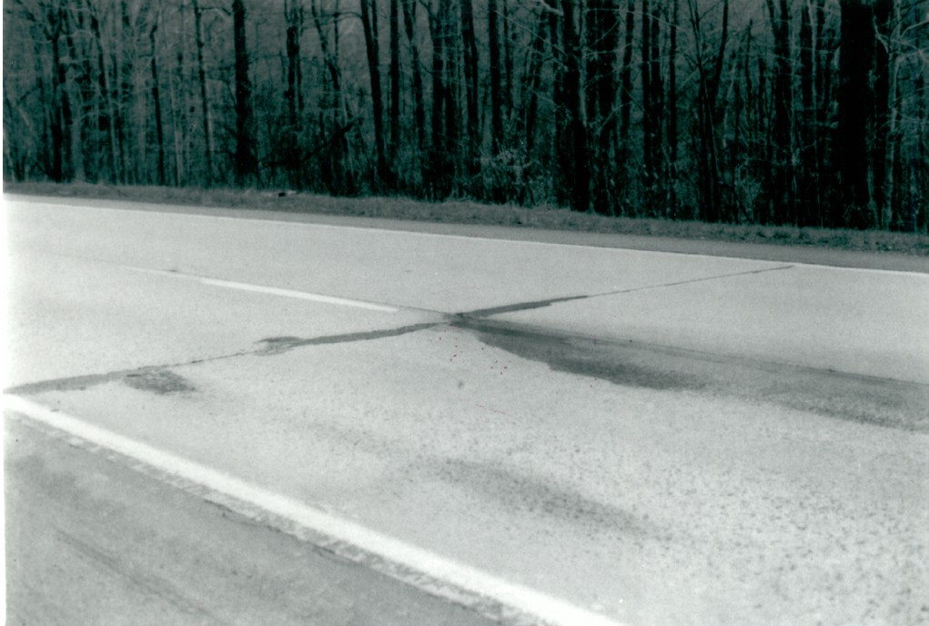
Figure 20. PCC Pavement (Water Pumping from Transverse Joint)
