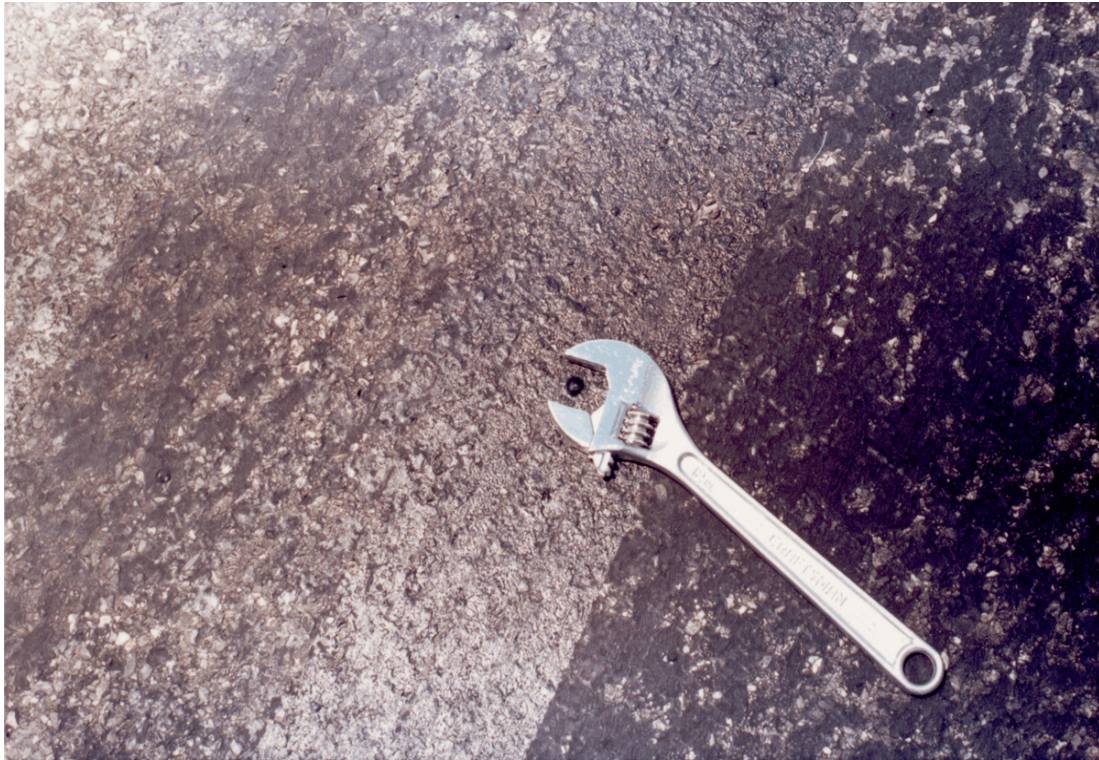
Figure 5. East-West Turnpike (Asphalt Bubbles - One Framed by Wrench)
