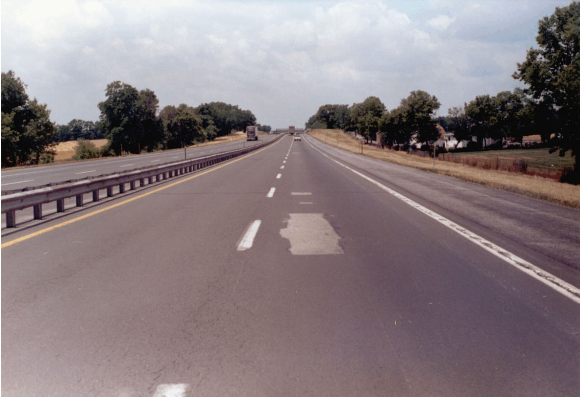
Figure 8. East-West Turnpike (Closeup of Patched Potholes)
