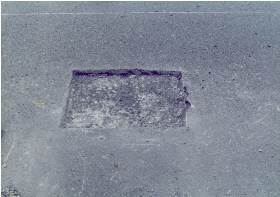
Figure 12. East-West Turnpike (Pothole After Removal of Wearing Course)
