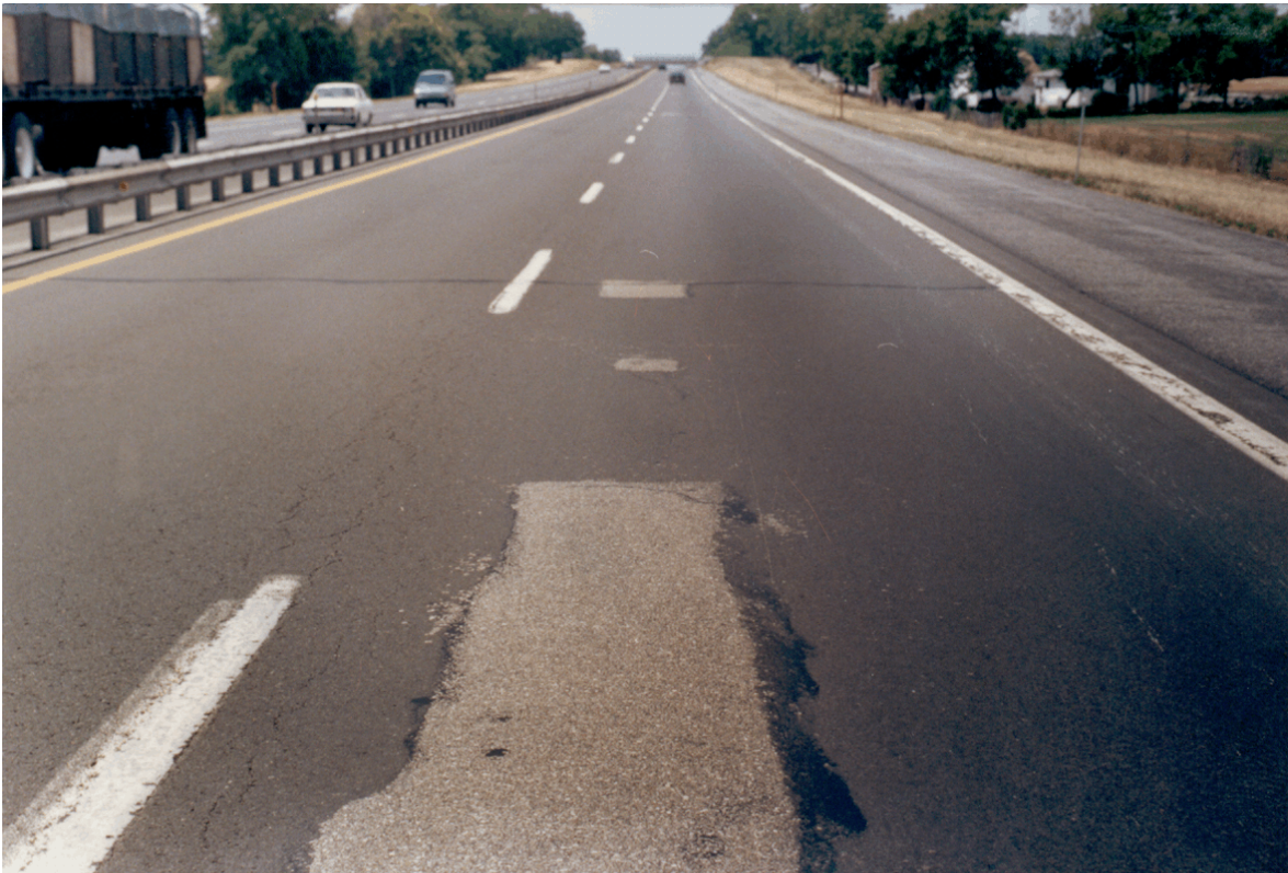
Figure 9. East-West Turnpike (Closeup of Long Patched Pothole)
