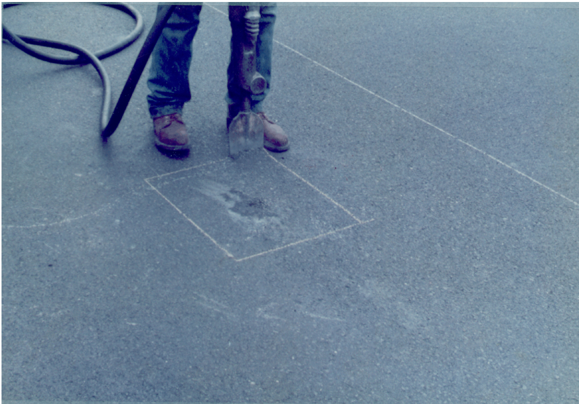
Figure 11. East-West Turnpike (Pothole with Rectangular Outline for Jack Hammering)
