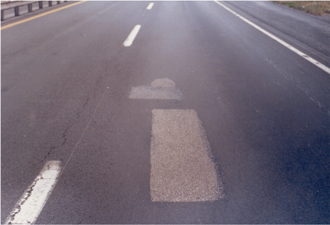
Figure 10. East-West Turnpike (Potholes Patched at Different Times)
