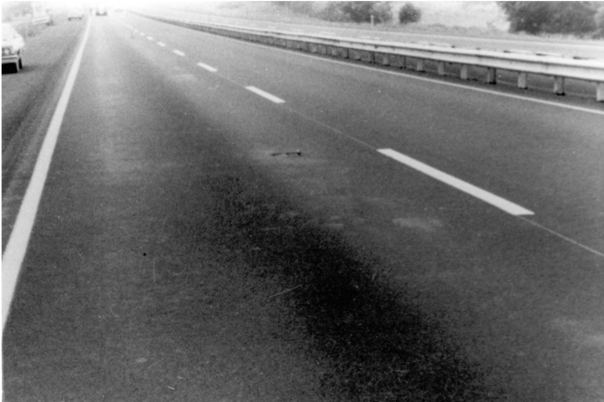
Figure 3. East-West Turnpike (General View Showing a Typical Pothole)
