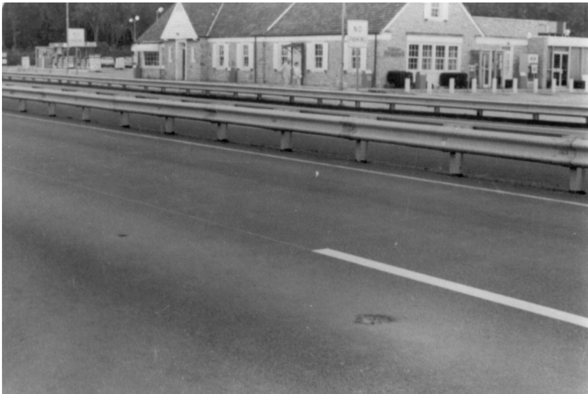
Figure 4. East-West Turnpike (Closeup of Potholes in Inside Wheel Track)
