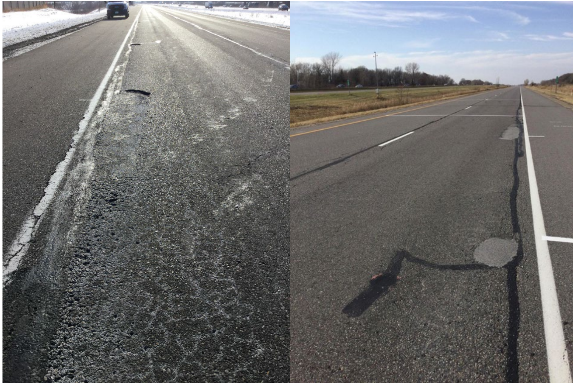
Figure 13 Cell 18 Potholes along Longitudinal Construction Joint in 2020
