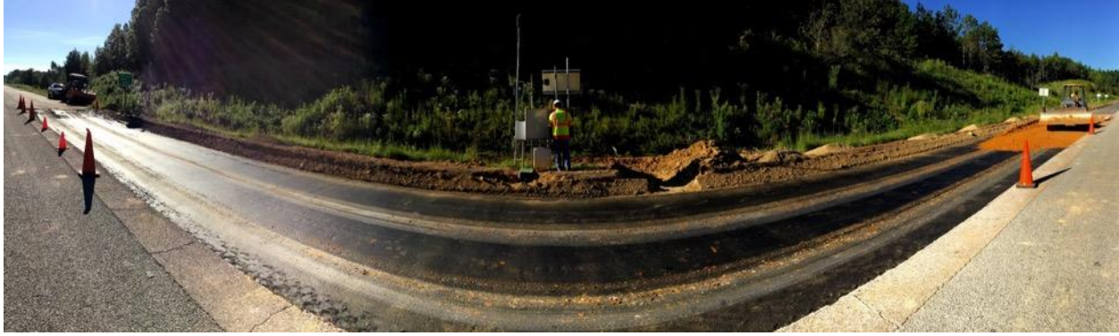
Figure 6. Placement of Silty-Sand Base on Prime Coated LTS in Section S2 (Panorama Image)
