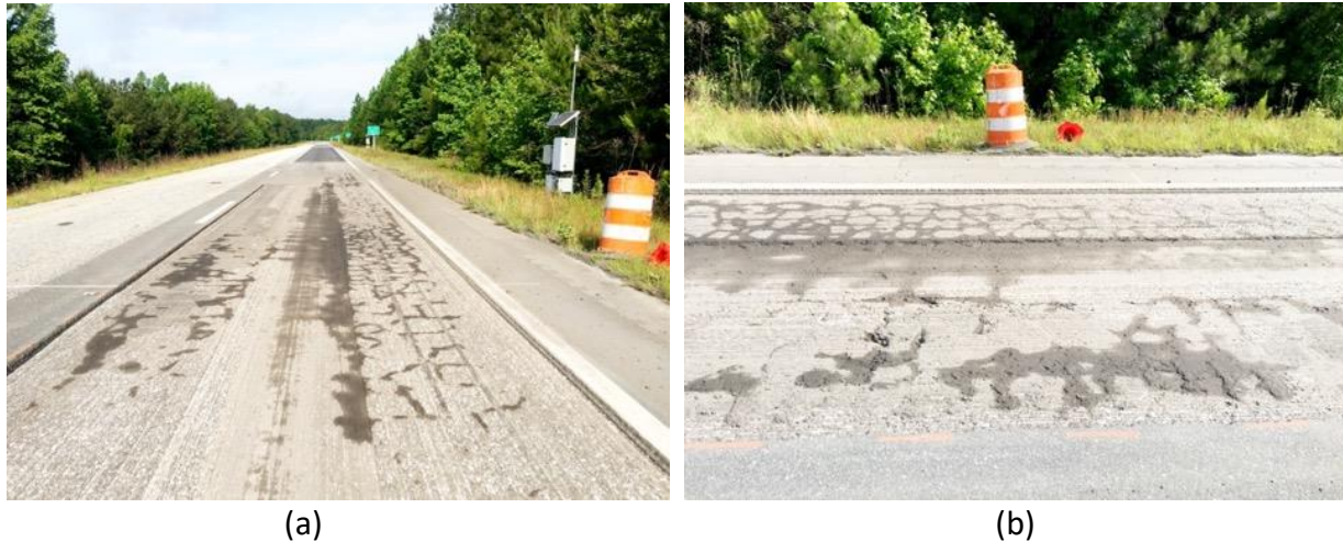
Figure 7. Section N7 Milled and Inlaid in May of 2020 (a) Milled Surface Showing Bottom-Up Cracking (b) Area of Severe Bottom-Up Cracks
