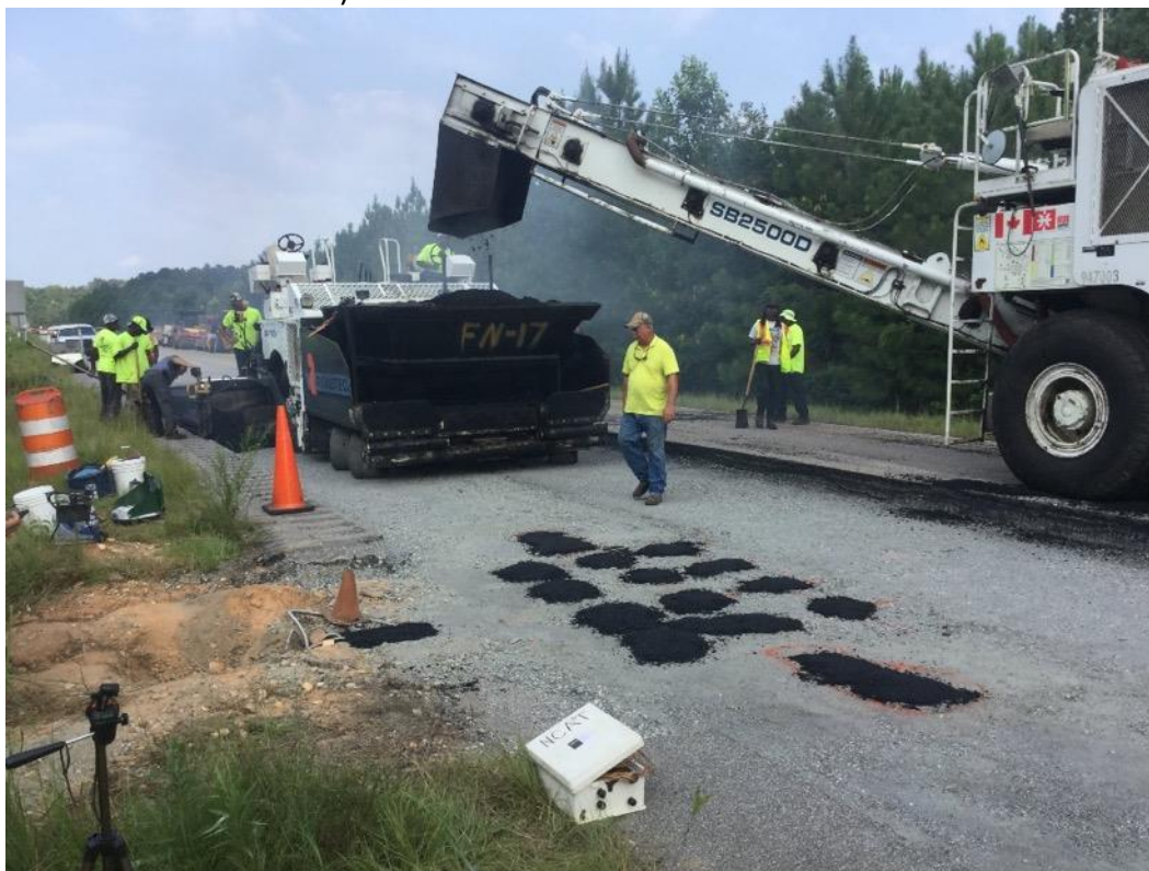
b) Gauges Covered with Sieved Mix Before Paving Figure 3. Instrumentation Prior to Paving
