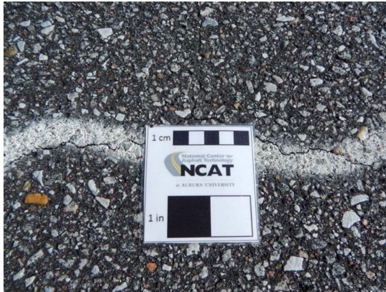
Figure 4. Close-up of Hairline Cracks in Sections N7 and N1
