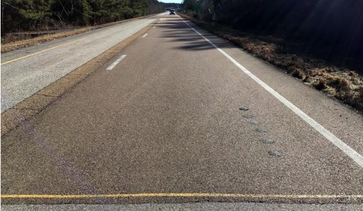
Figure 12. Section S2 Near the End of Trafficking
