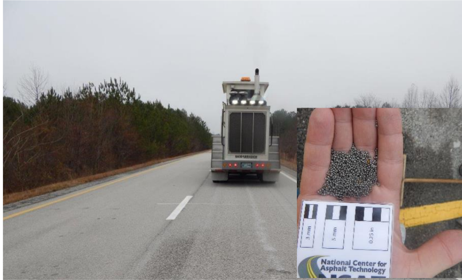
Figure 29. Application of Shotblasting Treatment to S7A and S7B and Close up of Steel Shots
