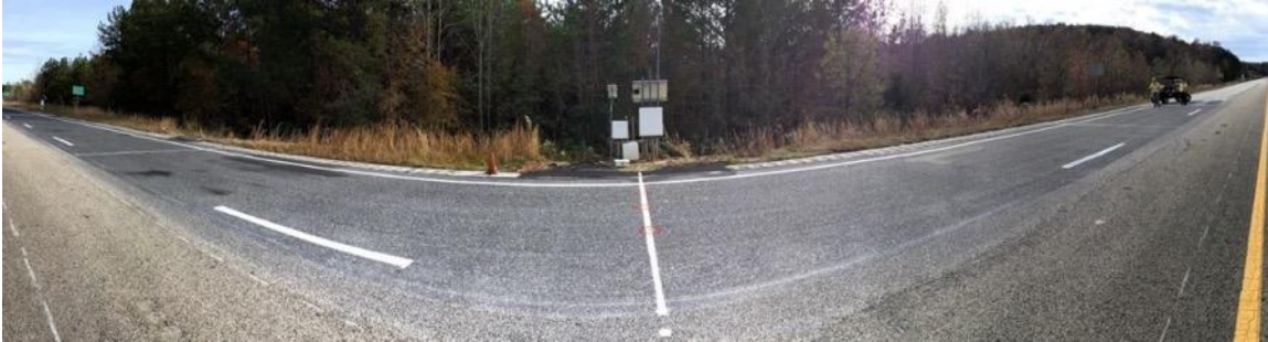
Figure 6. Section S9 After Grinding
