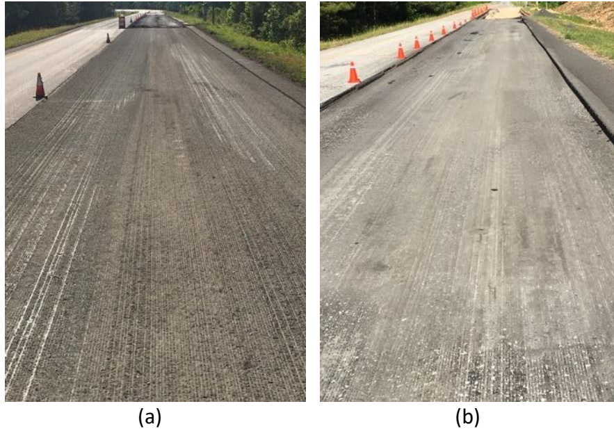
Figure 3. Existing Pavements after Milling in (a) Section N9 and (b) Section S1
