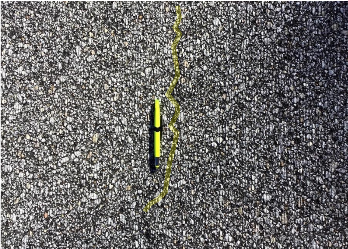
Figure 11. Section S9 Longitudinal Crack at Edge of Inside Wheelpath
