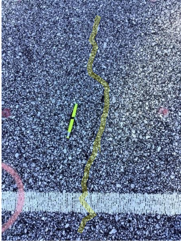
Figure 10. Section S9 Longitudinal Crack at Edge of Outside Wheelpath
