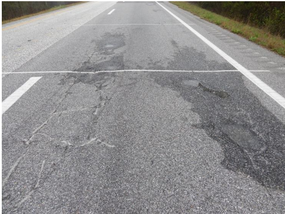
Figure 5. Cracking and Depressions in Untreated Section
