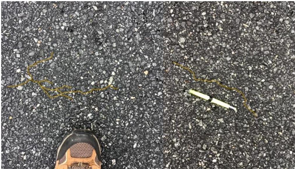
Figure 2. Sample Cracking in N4-4"AC on 1/25/2021 (29.6 Million ESALs)
