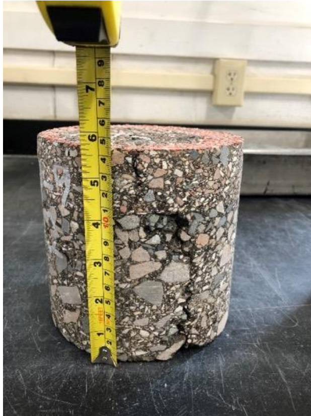
Figure 20. Field Core from Cracked Area in Section N9
