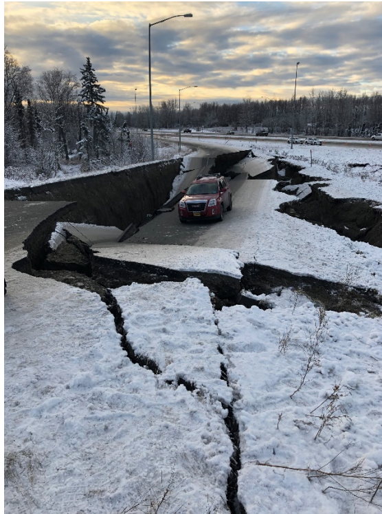
Figure 7. Failed Section of Minnesota Drive Ramp after 2018 7.0 Alaska Earthquake ( Photo Credit Knik Construction )
