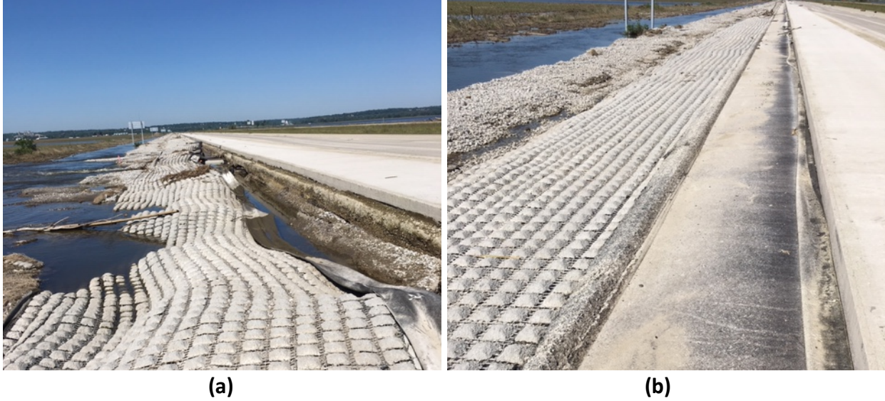
Figure 5. (a) Failed Grid Matting and (b) Asphalt Wedge Placed to Assist in Maintaining Mat Stability (Photo Credit Dr. Scott Schram, Iowa DOT)
