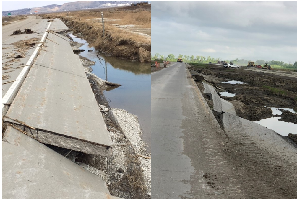
Figure 3. Shoulder Failures as a Result of Flood Water Undermining (Photo Credit Dr. Scott Schram, Iowa DOT)
