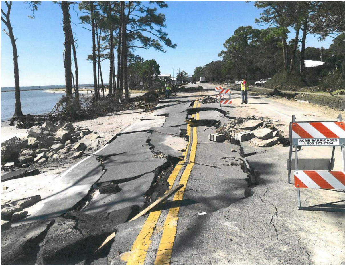
FIGURE A1. Hurricane Damage as A Result of Hurricane Michael on State Route 30 (US-98) in Franklin County Florida (Photo Credit Kevin Wall, Anderson Columbia)
