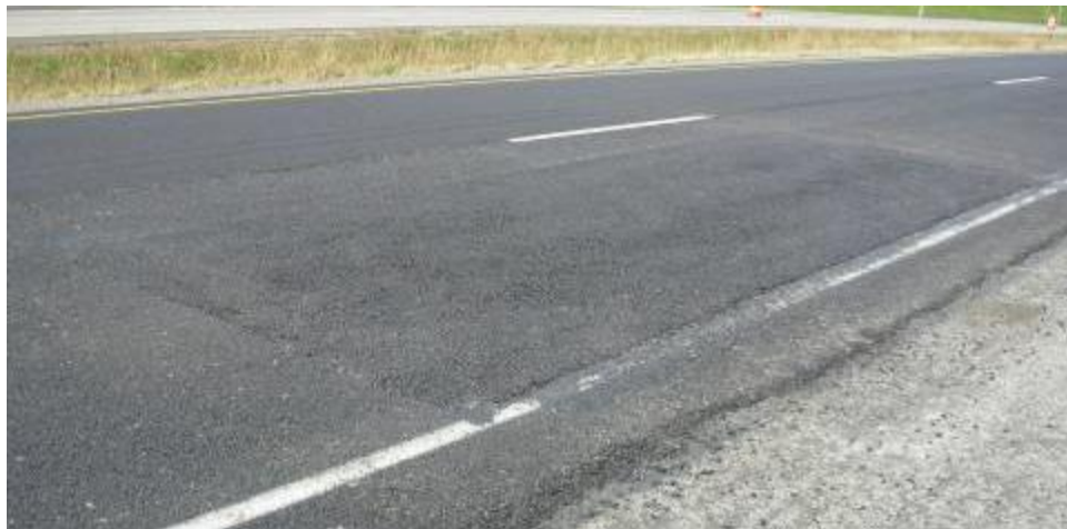
Figure 15. Patched Area Where Mix Placed in Cold Weather Had Raveled
