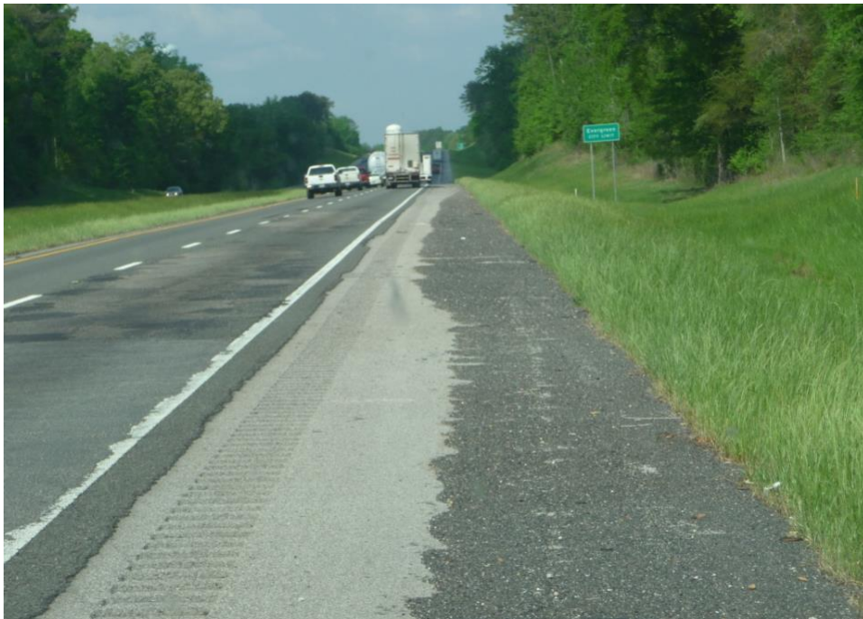
Figure 3. Loose Aggregate on Northbound Shoulder at Milepost 94.1 (near Evergreen)
