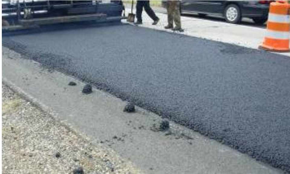
Figure 14. Cold Lumps Removed From OGFC
