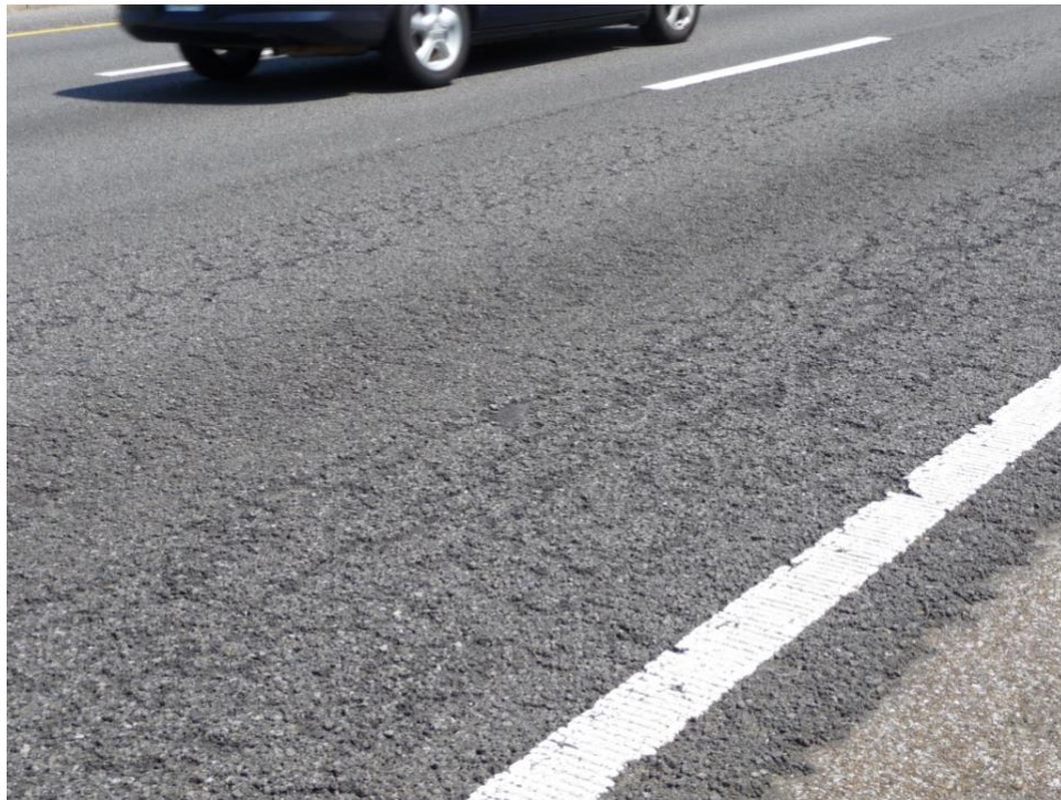
Figure 1. Raveling in Southbound Outside Lane at Milepost 93 (near Evergreen)
