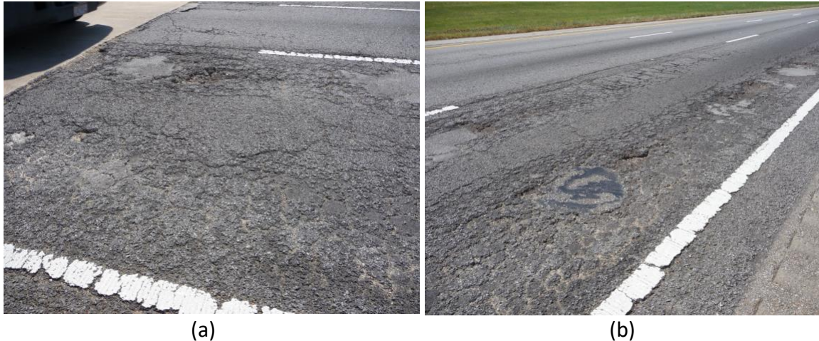
Figure 4. Failures on Northbound Outside Lane at Milepost 173 (Alabama River)
