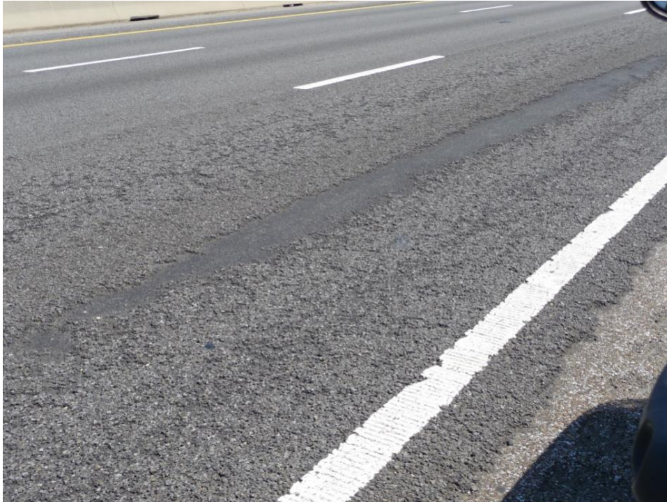
Figure 2. Raveling in Southbound Outside Lane at Milepost 177.9 (near Prattville)
