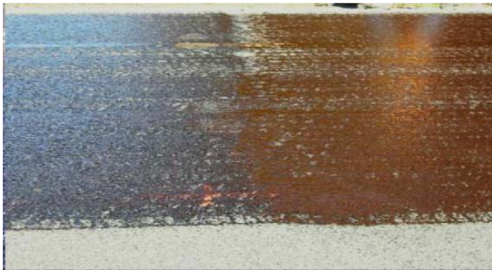
Figure 4. Broken and Unbroken Tack Coverage Over an Un-Milled Pavement Surface (Washington State DOT, 2003)
