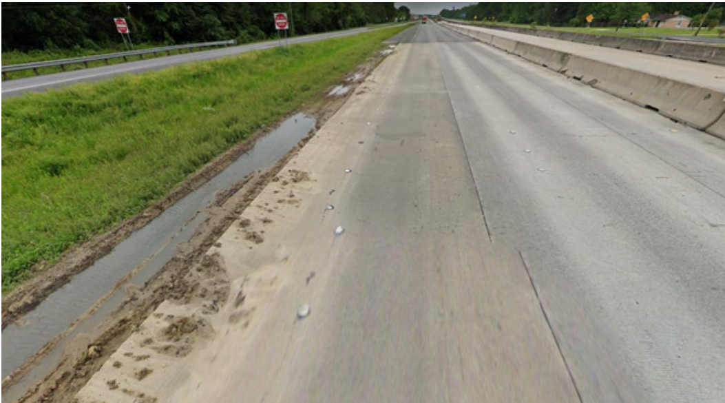
Figure 7. Excessive Drop-Off, I-10 Texas
