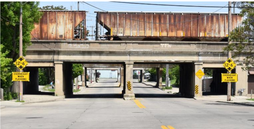
Figure 9. Inadequate Bridge Clearance, Location Unknown
