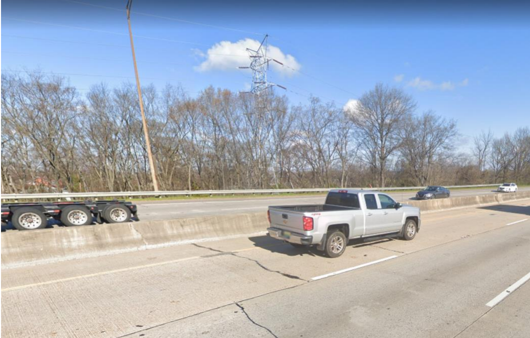
Figure 8. Inadequate Barrier Wall Height, I-85 Georgia
