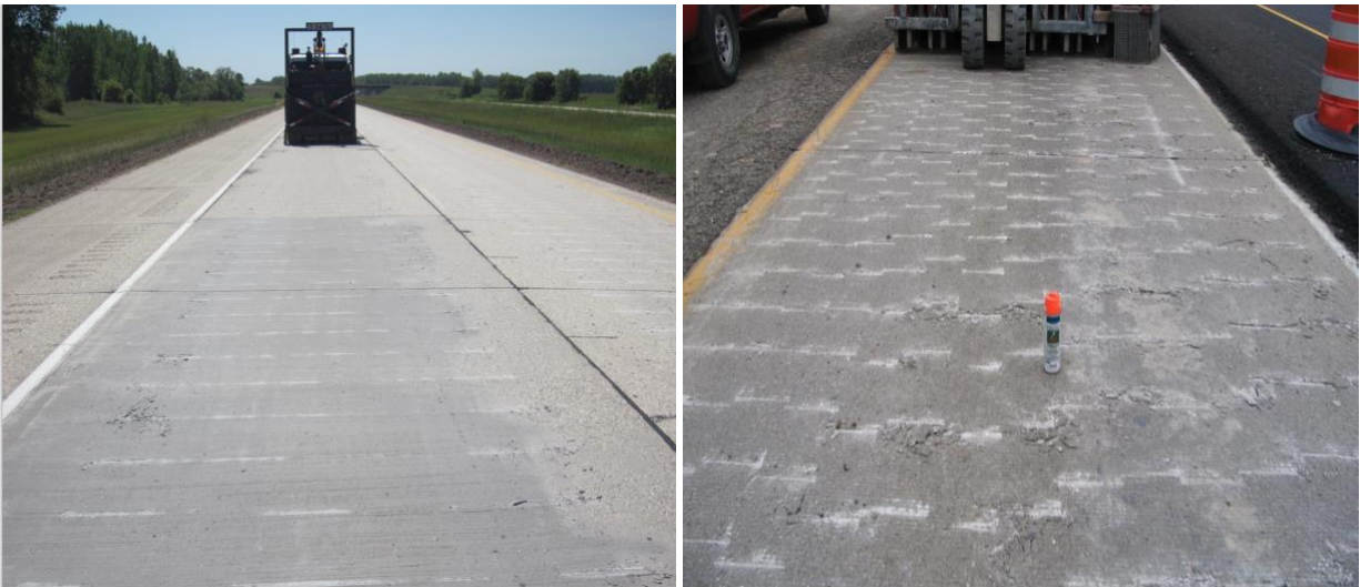
Figure 1. Typical Fractured PCC using C&S (left) and B&S (right) Methods (Antigo, 2019)
