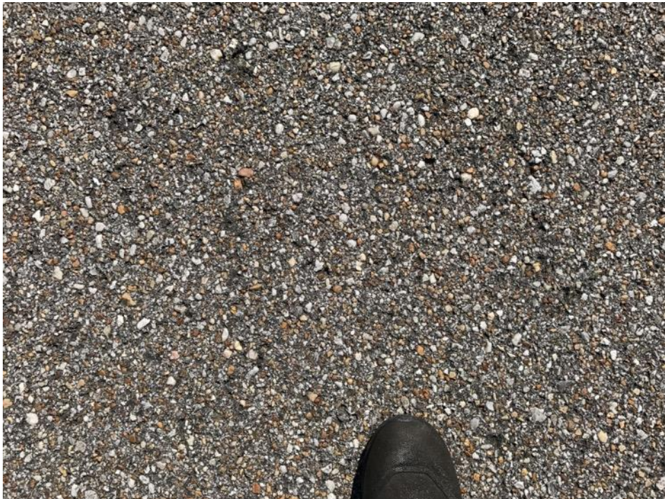
Figure 55 Example of Raveling Observed on US 80
