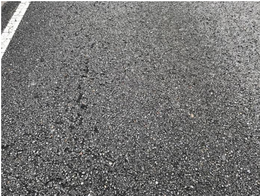
Figure 49 Close-Up View of Raveling on AL-35
