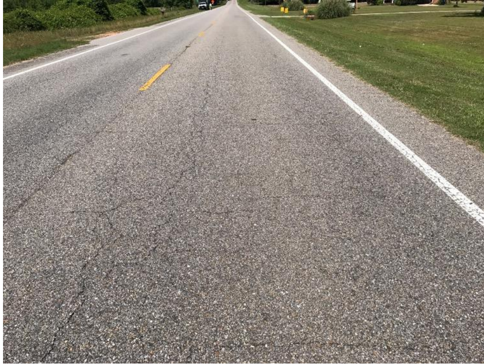
Figure 43 Fatigue Cracking in Wheelpaths Observed on US 29
