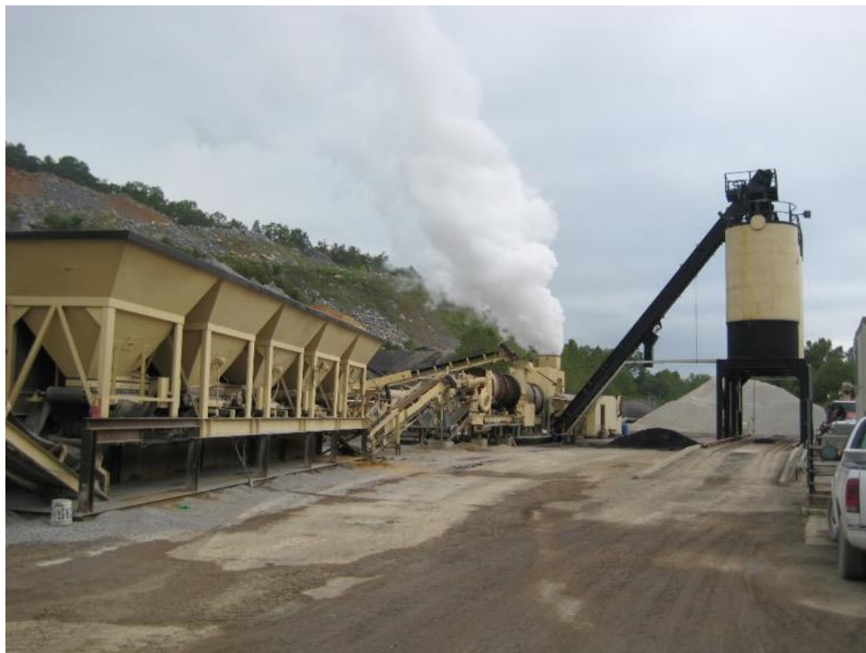
Figure 44 Good Hope Contracting’s ADM Plant in Collinsville, Alabama
