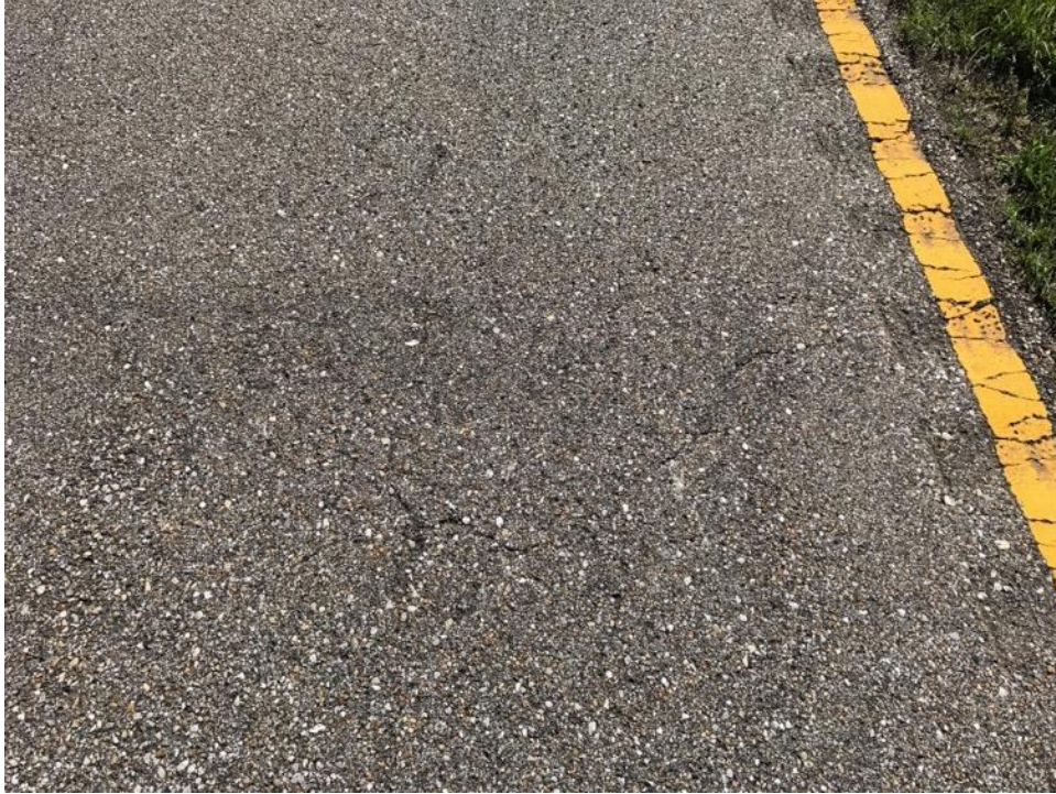
Figure 54 Low-Severity Cracking Observed on US 80
