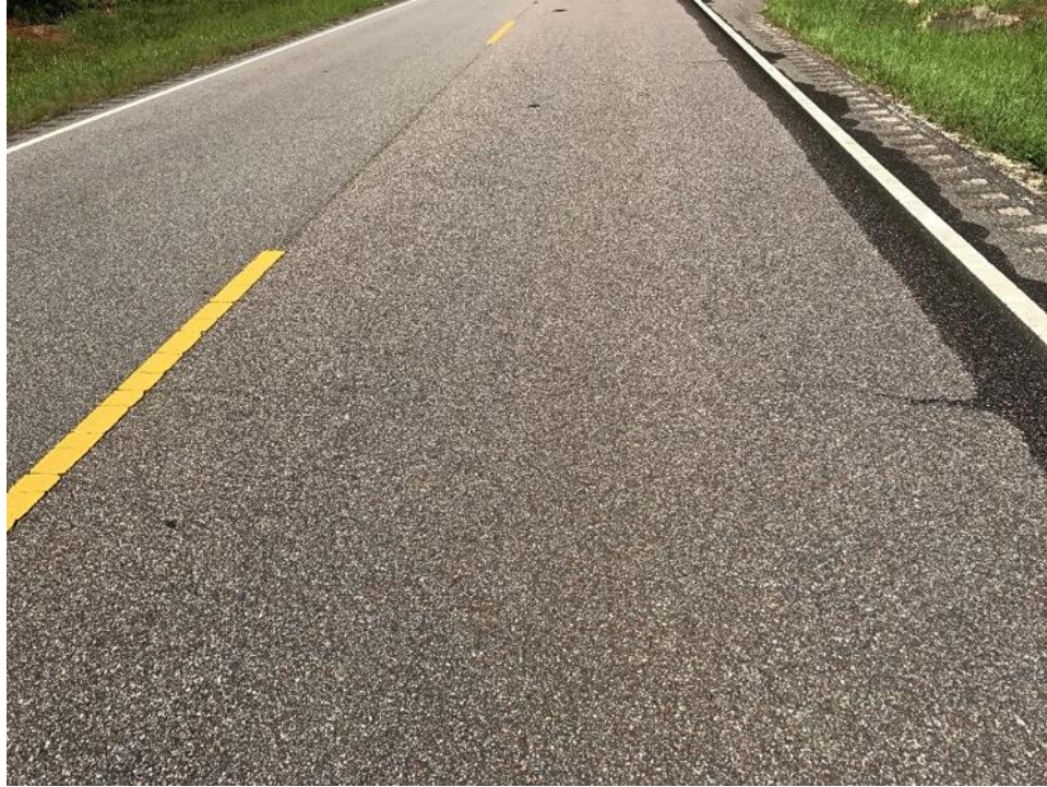
Figure 27 Low-Severity Transverse Cracking Observed on AL 50
