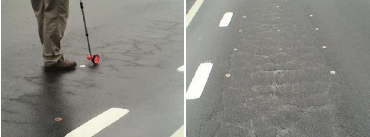
Figure 2 Examples of Bottom-Up Fatigue Cracking Observed at Pavement Surface.
