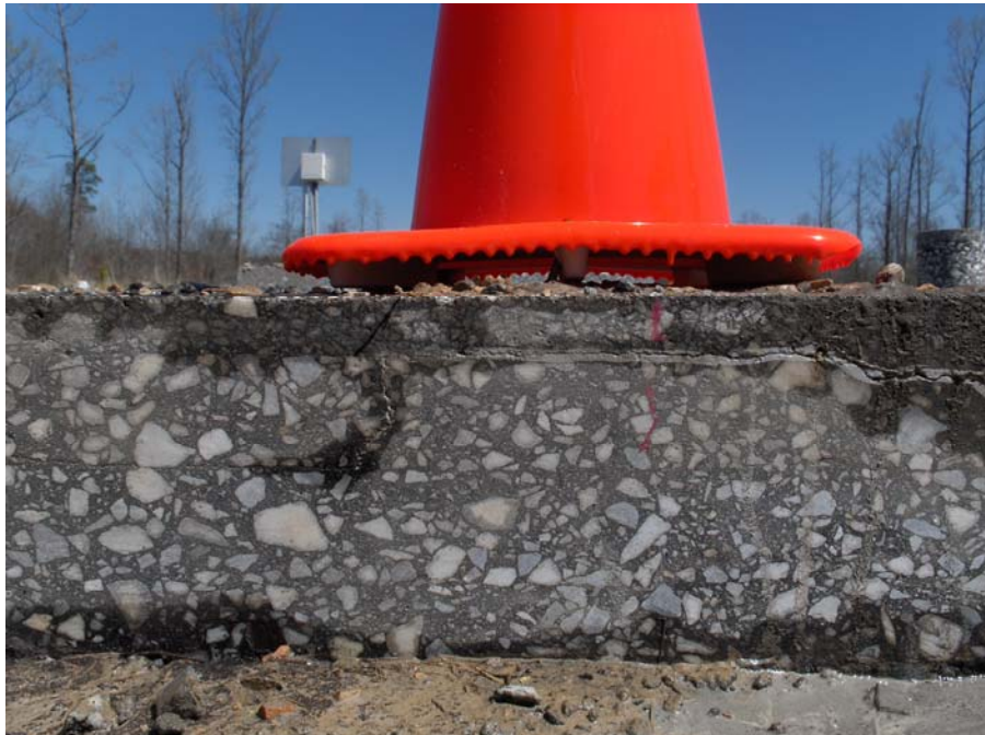
FIGURE 1 Delamination in HMA Pavement (11).
