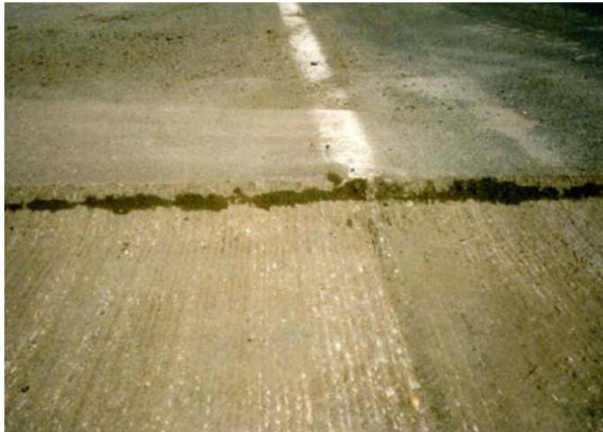
FIGURE 5 Moisture Present at Delaminated Interface between HMA Layers (12).
