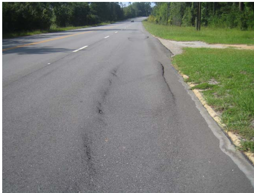
FIGURE 3 Slippage Failure Due to Inadequate Bond.
