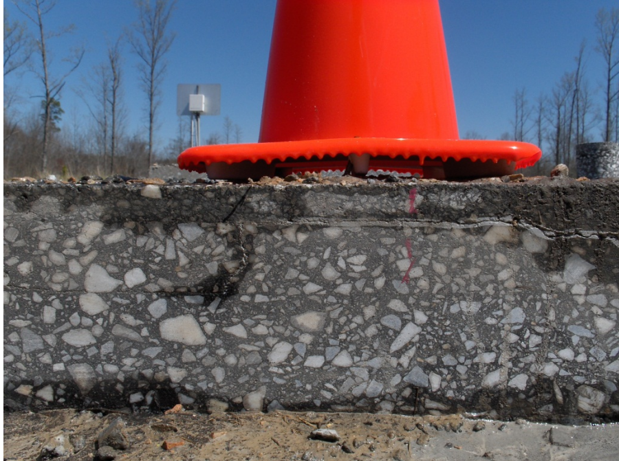
Figure 1 Delamination in HMA Pavement (II)
