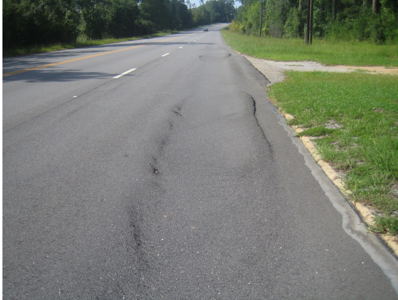
Figure 3 Slippage Failure due to Inadequate Bonding
