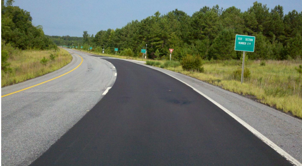
FIGURE 26 Rich Spot near the End of the HMA Control Test Section
