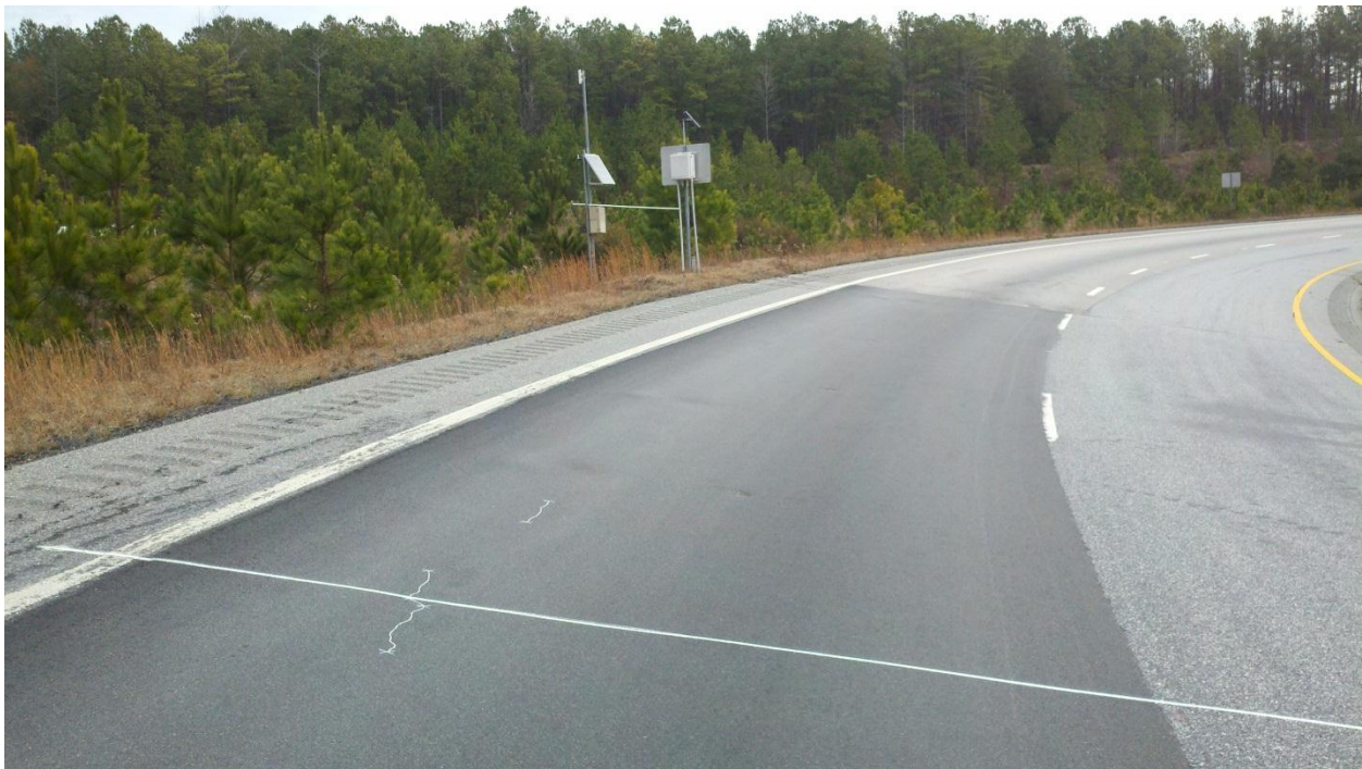
FIGURE 29 Cracking Observed in the Control HMA Test Section
