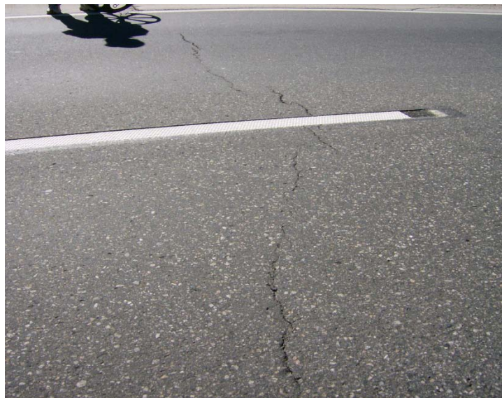
Figure 16 Example of Transverse Crack in WMA Test Section
