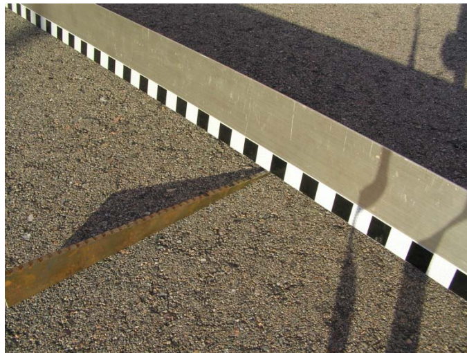
Figure 15 Example of Rutting in WMA Test Sections
