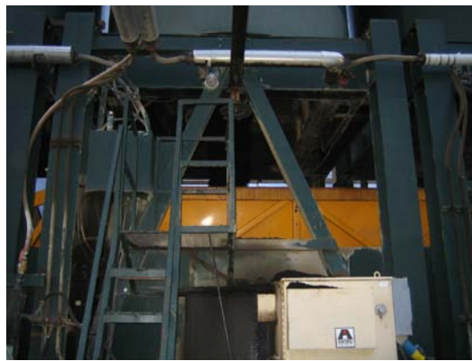
Figure 9 No Visible Smoke or Fumes from Sasobit WMA Production at the Plant
