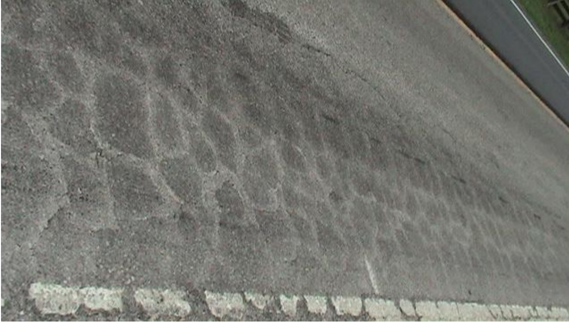
FIGURE 4 Pavement Distress Under Evotherm DAT Lift
