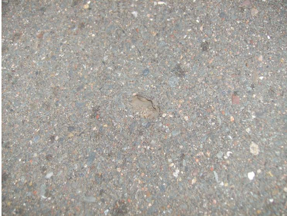
FIGURE 8 Coarse Aggregate Pop-out from Sasobit ® Test Section.
