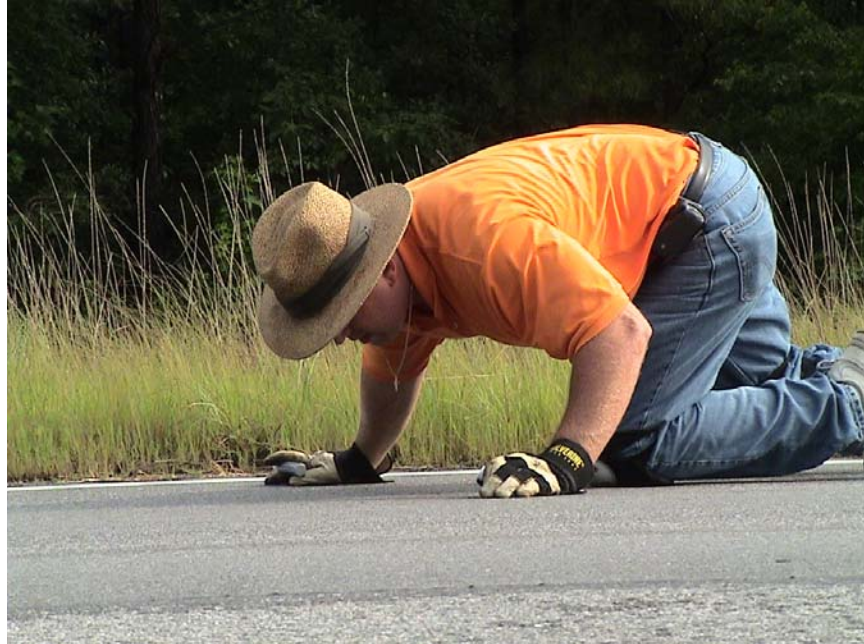
FIGURE 46 Crack investigation technique (12).
