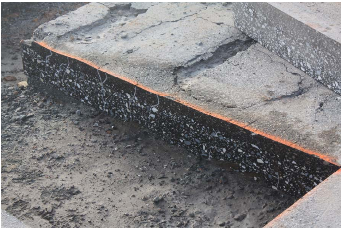
FIGURE 2 Fatigue cracking on a roadway.
