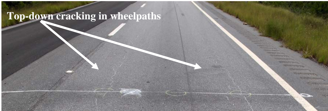
Figure 2.2. Top-Down Cracking in Section N5
