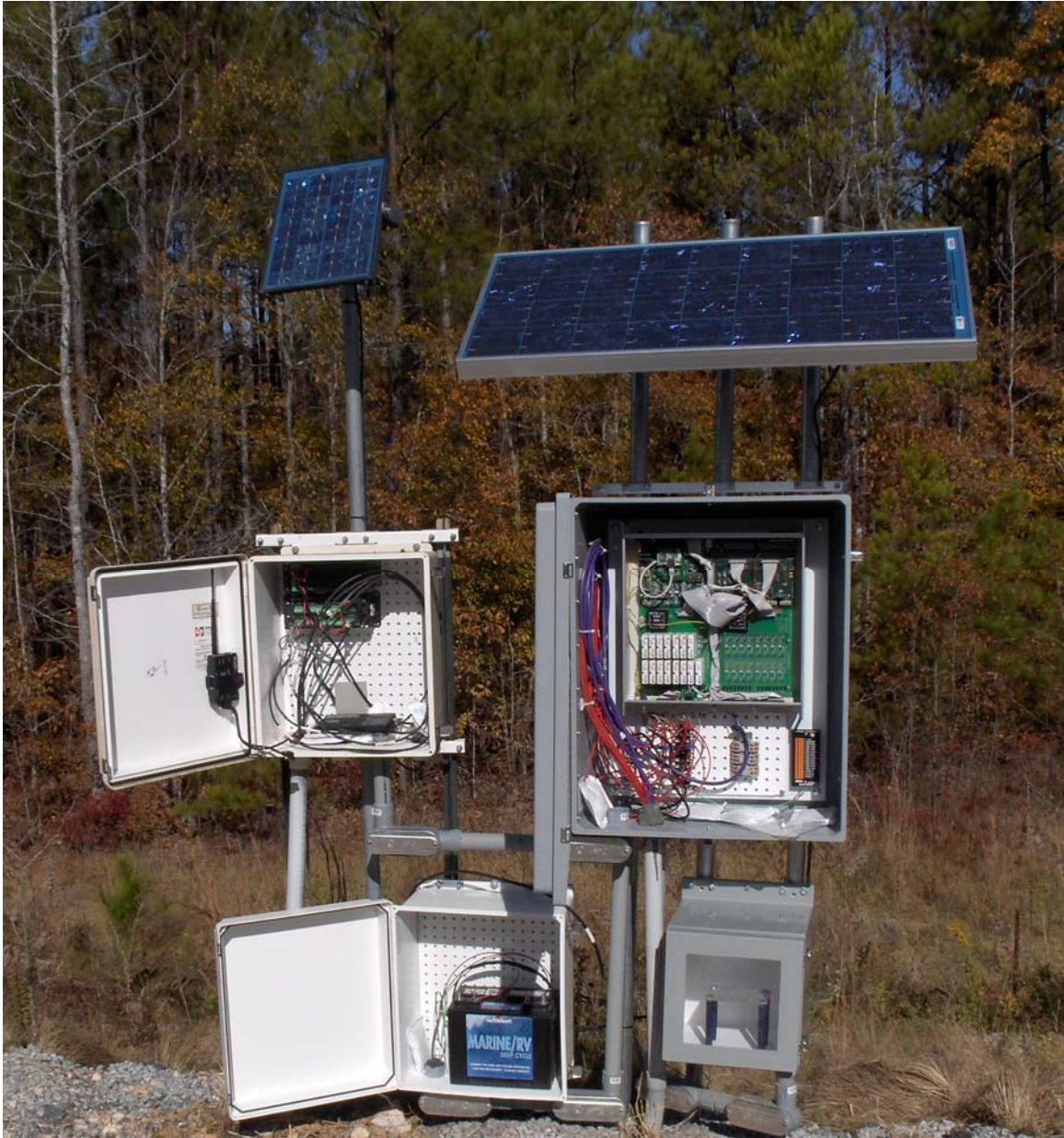
Figure 3.16. Roadside Data Acquisition Enclosures and Equipment
