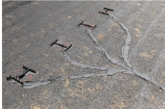
a. Gauges Laid Out with Sand Asphalt Tack under Gauges and Covering cables.
