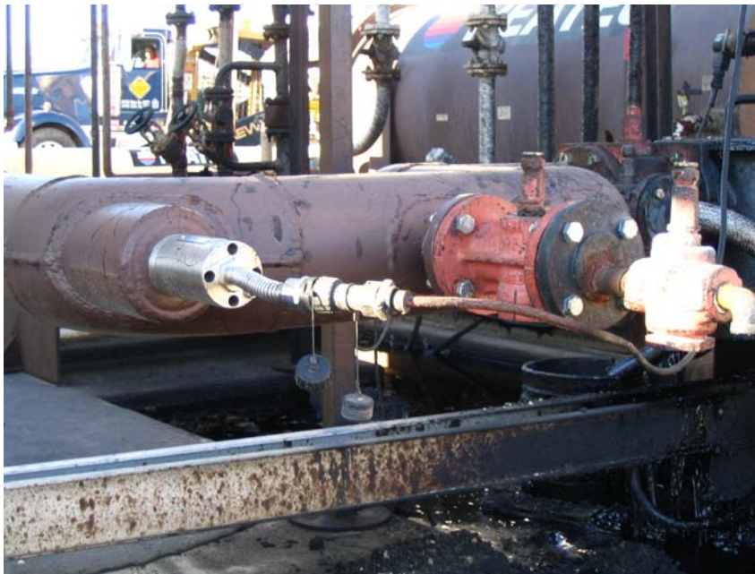
FIGURE 5. In-Line Viscometer Installed in the Asphalt Supply Line.
