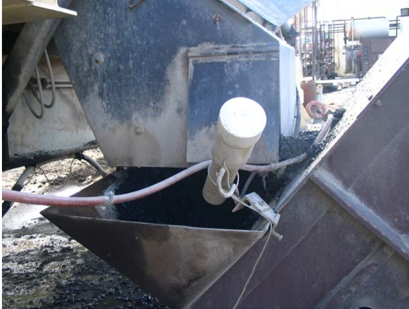
FIGURE 6. Infrared Temperature Sensor at Drum Discharge.
