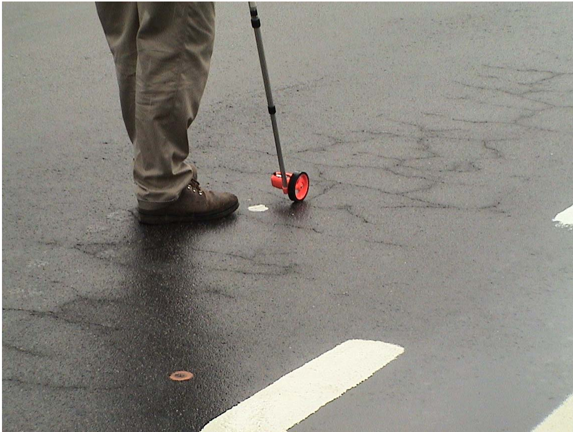
Figure 5.17 First Observed Fatigue Cracking on Section N1.
