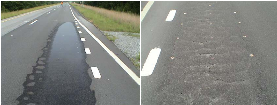
Figure 2.12 Pavement Drainage and Pumping Problems.
