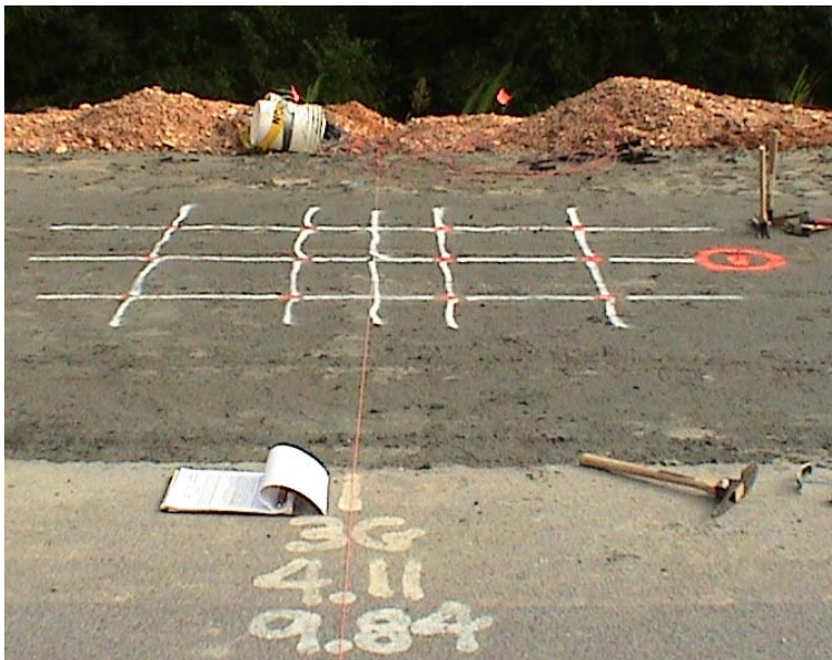
Figure 4.9 Gauge Location Markings for Cell N3.
