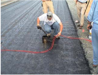
b) Tacking Gauge Cables
