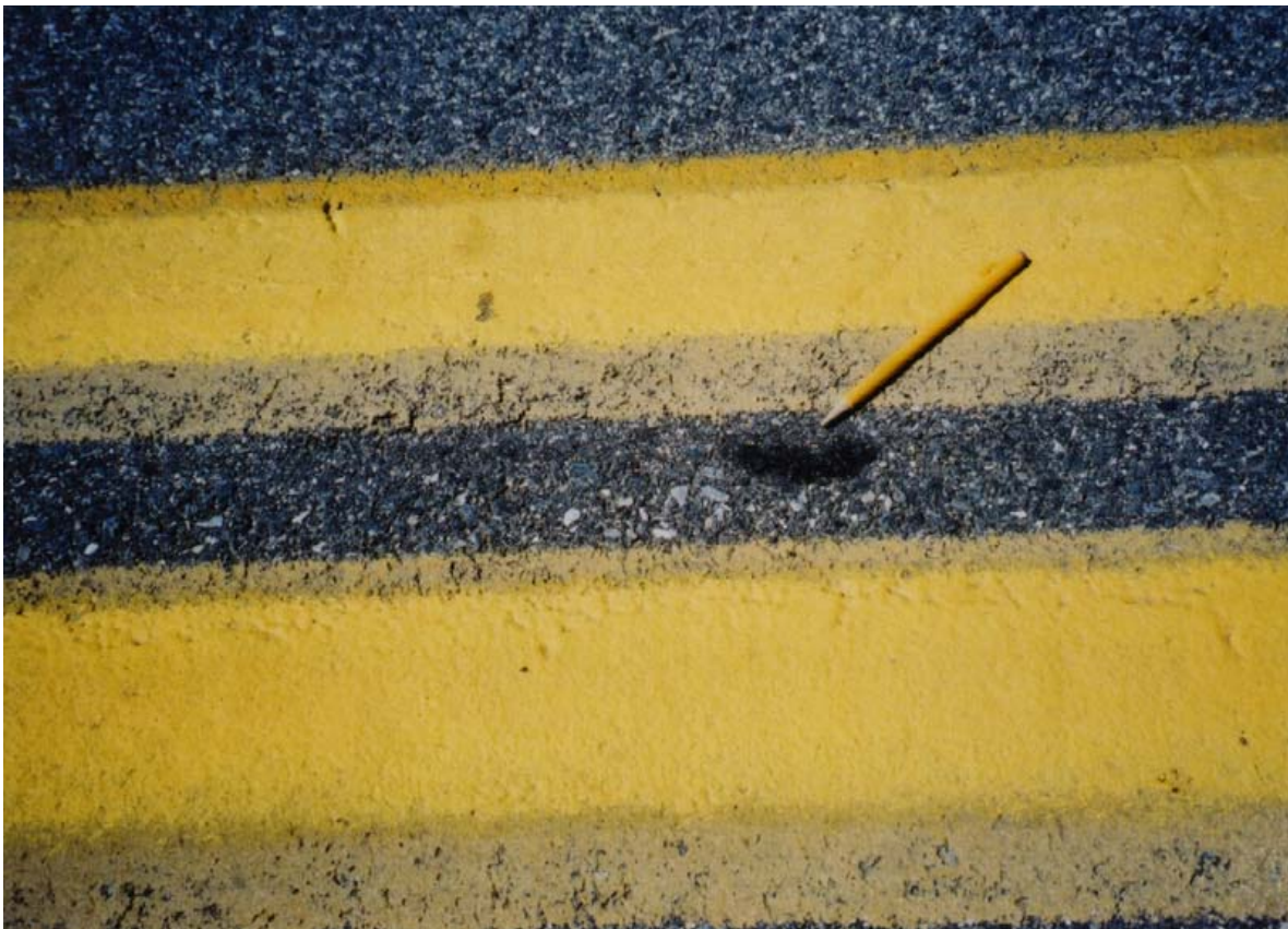
Figure 6. Closeup of Joint with Rubberized Asphalt Tack Coat, Joint Between Yellow Stripes Is Hardly Visible, Pencil Pointing to Excess Tack Coat on the Surface in a Few Spots Helped Locate the Joint
