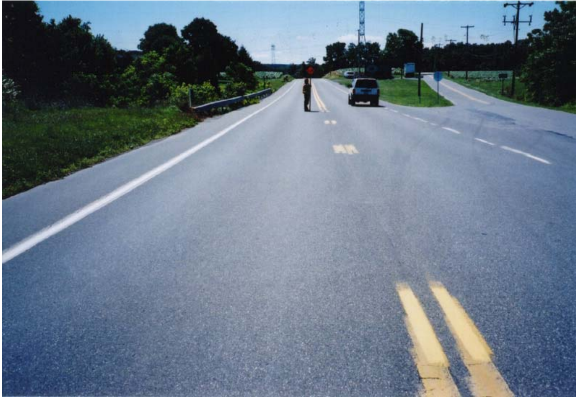
Figure 7. General View of Section Where Cutting Wheel Used, No Significant Cracking Can Be Seen, Joint Not Visible in Most of the Section
