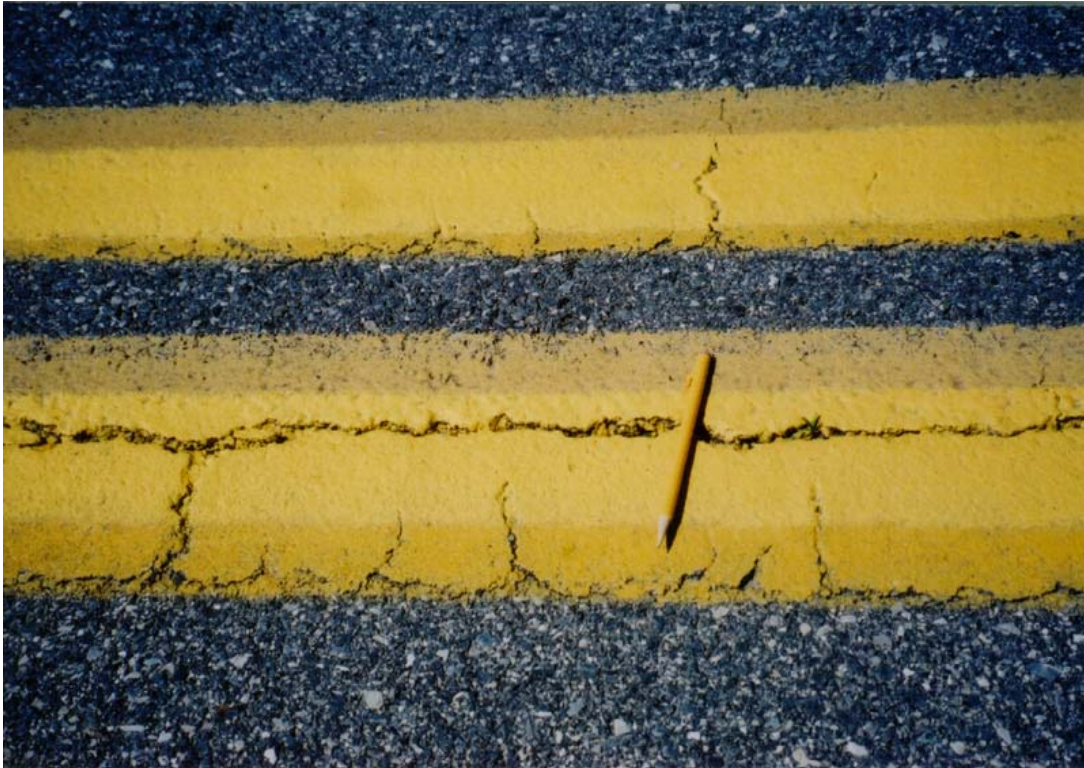
Figure 11. Closeup of Jagged Cracking in the Section Rolled from Cold Side, the Crack Is Generally Wider and Deeper than That in Section Rolled from Hot Side
