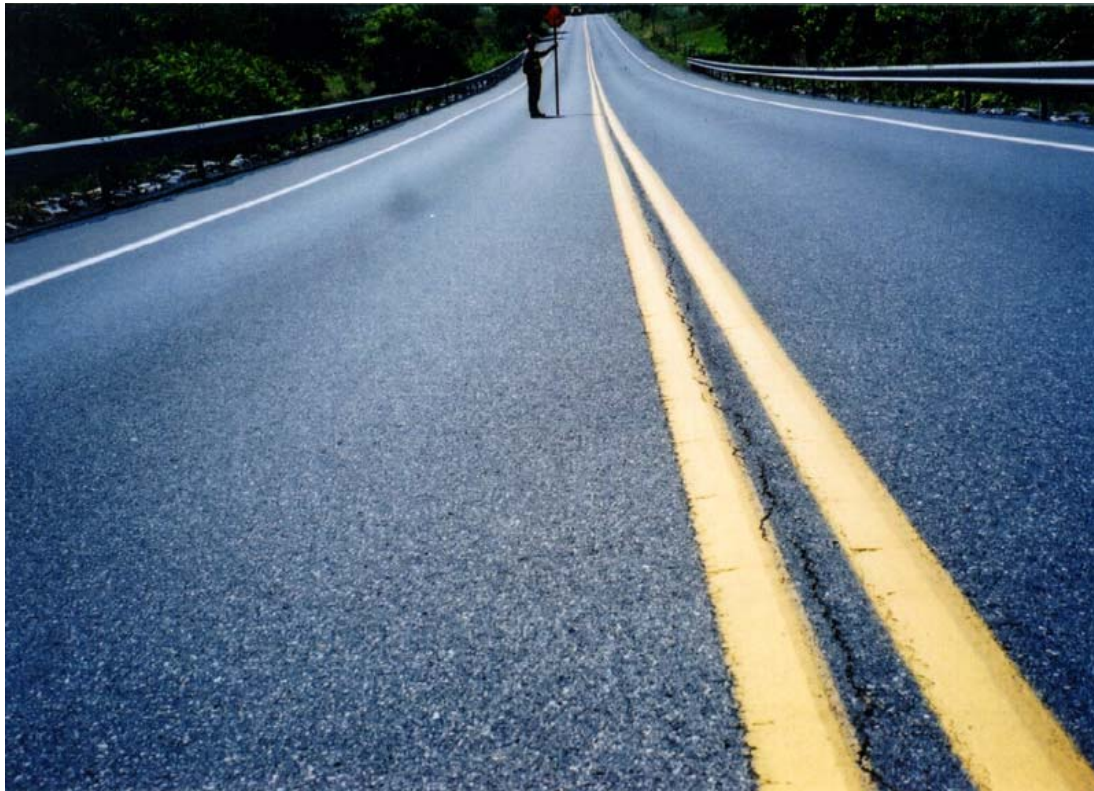
Figure 10. Section Where Rolling Was Done from Hot Side with 152 Mm Overlap on Cold Side, a Jagged Crack Can Be Seen Between the Yellow Stripes
