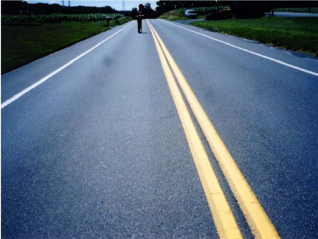
Figure 8. General View of Section Where Rolling Was Done from Hot Side 152 Mm Away from the Joint, No Significant Cracking Can Be Seen, Joint Visible in Most of the Section
