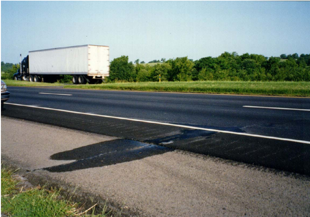
Figure 18. Water Coming out of Thermal Cracks
