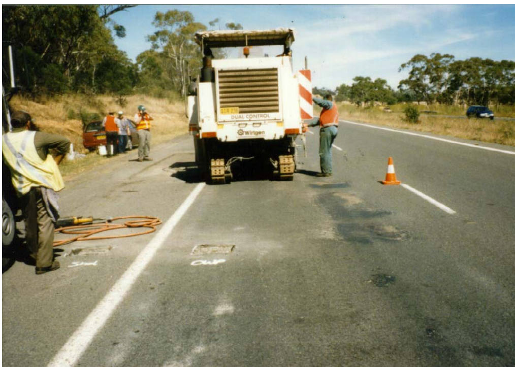
Figure 25. Potholes in the Southbound Slow Lane of Hume Highway (Another Location)
