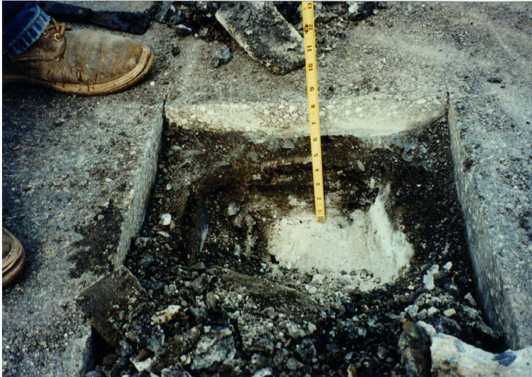
Figure 6. Hole Exposing All Asphalt Concrete Layers and PCC Surface at MP 217.65
