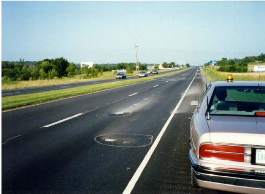
Figure 16. Potholing in the Inside Wheel Track of Slow Lane
