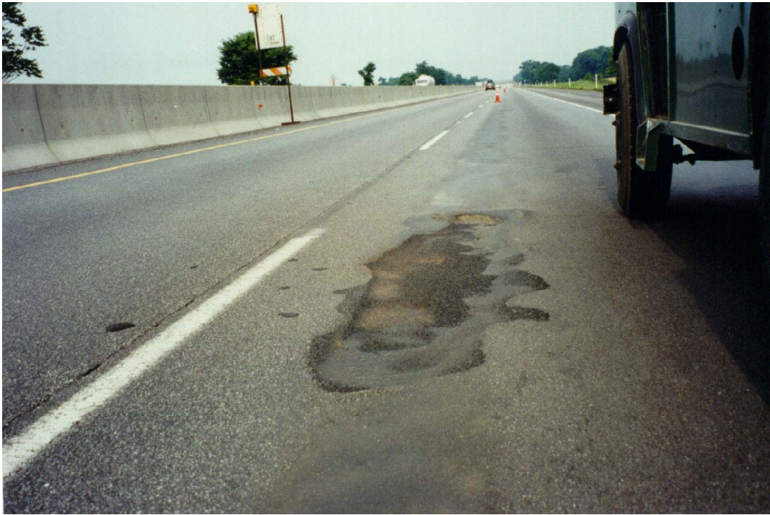
Figure 3. Potholes and Rutting in the Westbound Slow Lane Near MP 217.65
