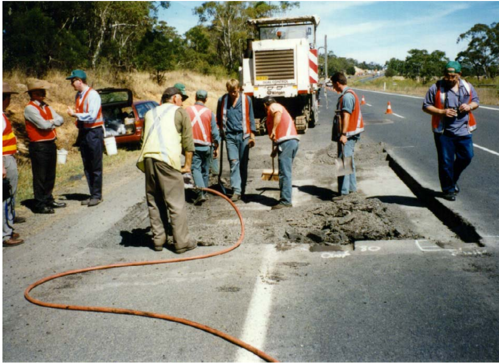
Figure 31. Cold Milling in the Slow Lane and Shoulder Area to Evaluate the Condition of Asphalt Layers
