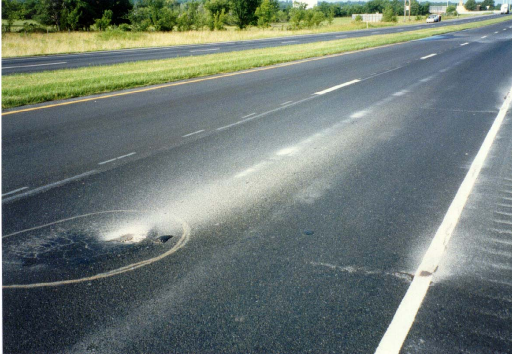
Figure 20. Big White-Stained Patches Near Potholed Areas
