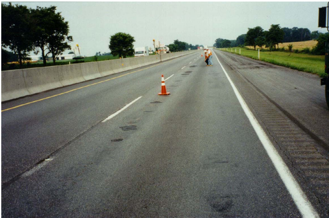
Figure 2. Potholes in Both Wheel Tracks of the Distressed Westbound Slow lane Near MP 217.65 (Most Potholes in the Inside Wheel Track)
