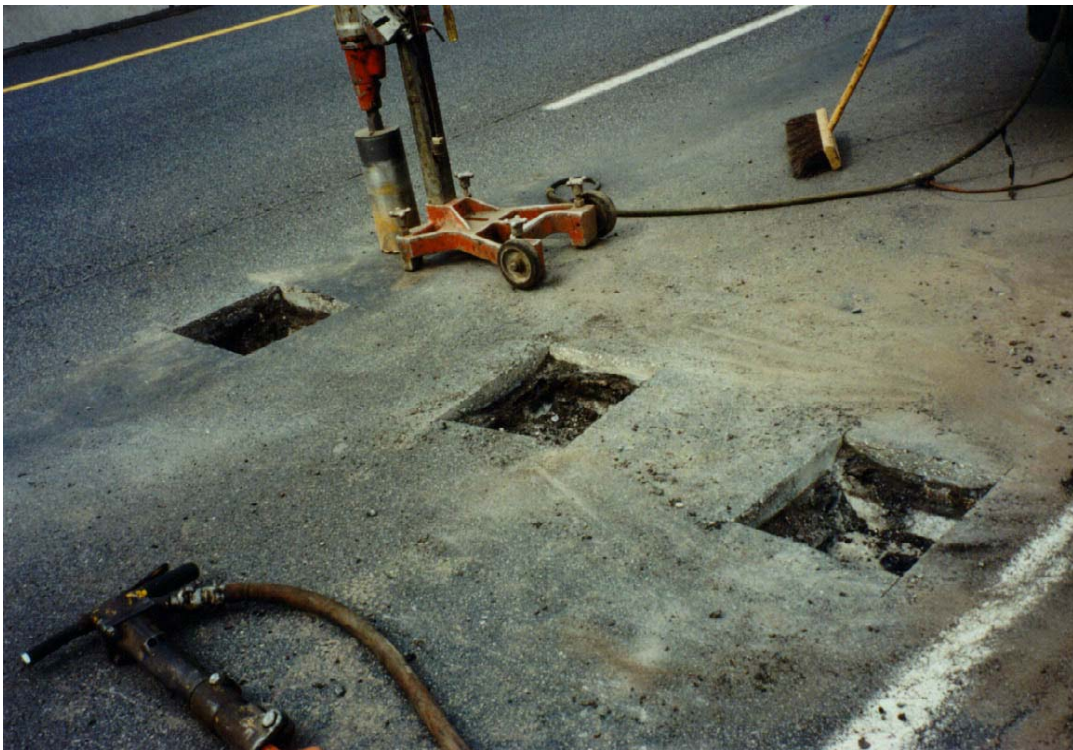
Figure 4. Three Square Holes Cut in the Westbound Slow Lane at MP 217.65
