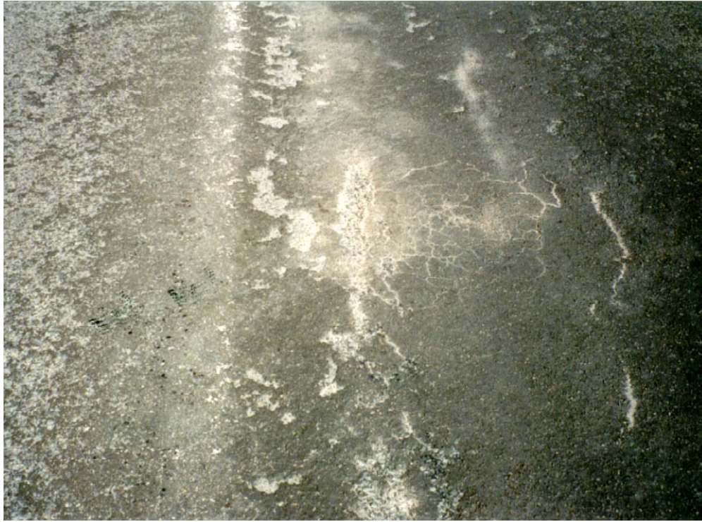
Figure 26. Stages of Pavement Distress: White Stains, Alligator Cracks, and Pothole
