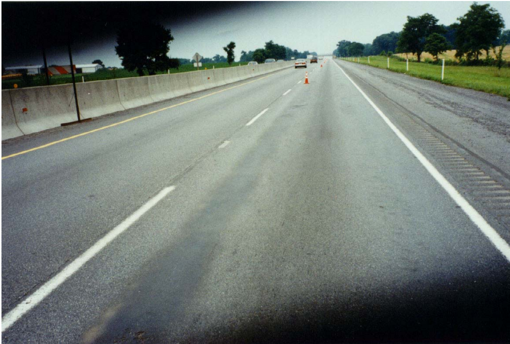
Figure 1. General View of the Distressed Westbound Lane Near MP 217.65 Showing Mud Stains, Flushing, and Potholes
