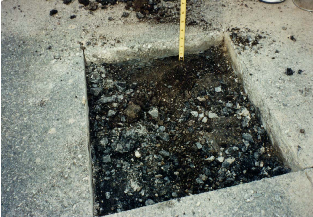
Figure 5. Hole Exposing New Gravel Wearing Course and Underlying Old Limestone Binder Course at MP 217.65
