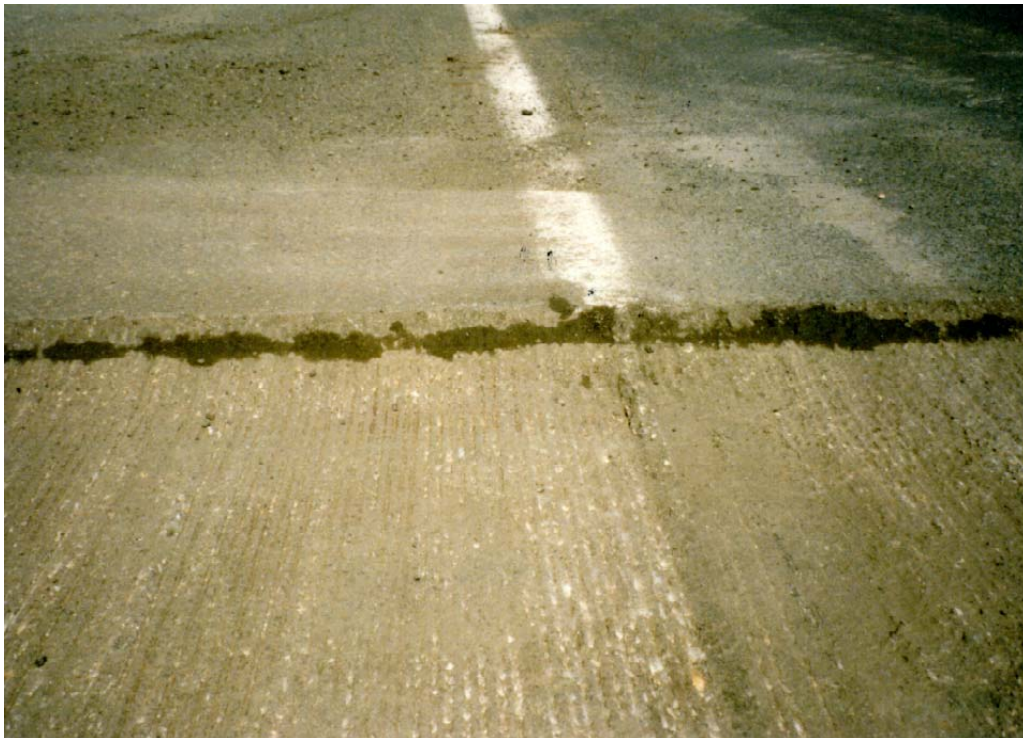
Figure 32. Wet AC 14 Course Just Below OGFC at the Edge of the Milled Trench
