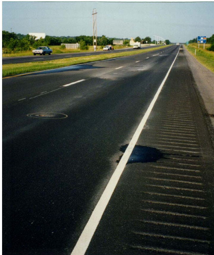
Figure 17. Potholes in the Inside Wheel Track of slow Lane (Another Location)
