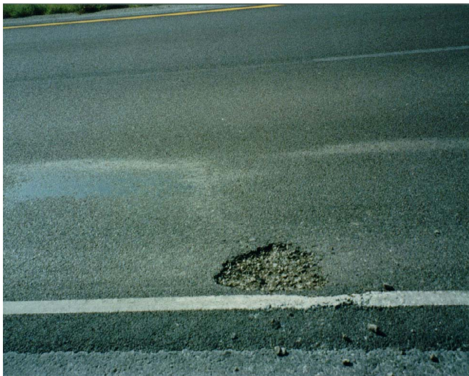
Figure 13. Three Stages of Stripping: White Stains, Flushing, and Pothole (I-40)
