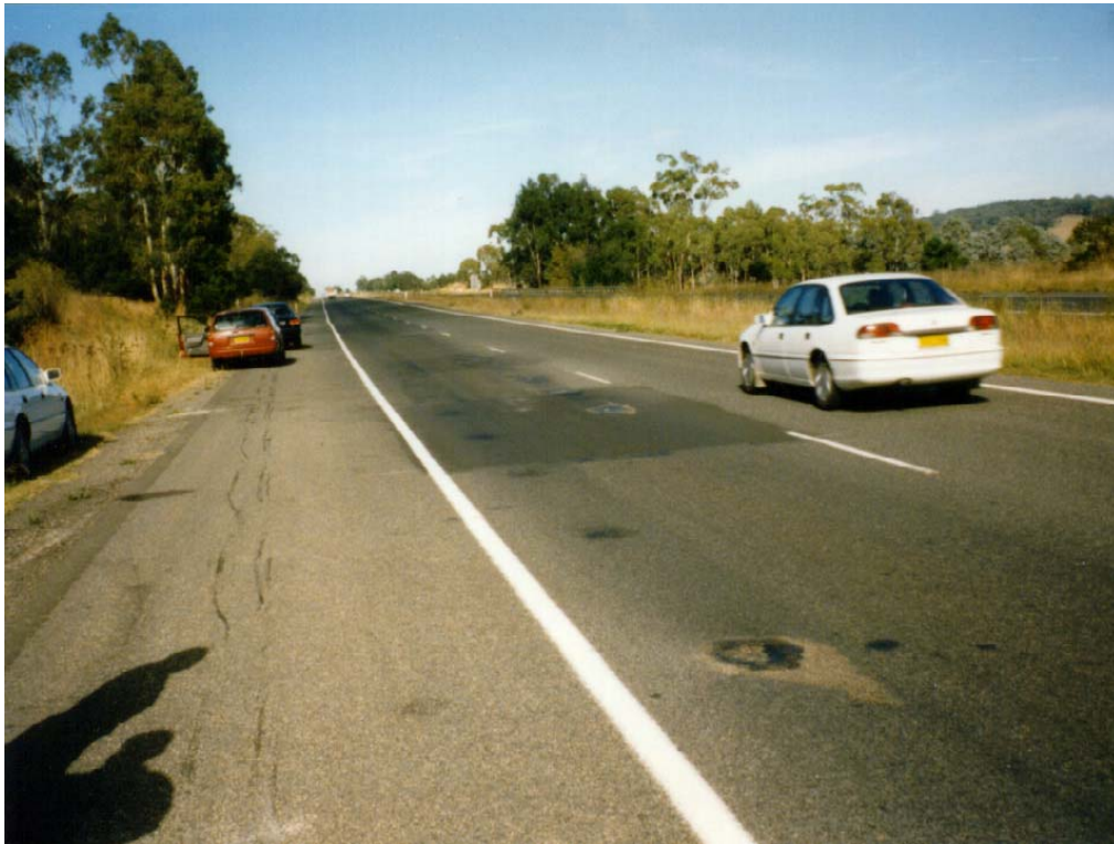
Figure 24. Pattern of Potholes and Patch Repairs in the Southbound Slow Lane of Hume Highway
