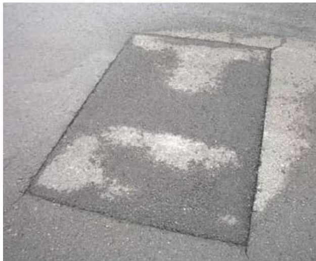
Figure 18. Patching and Utility Cut
