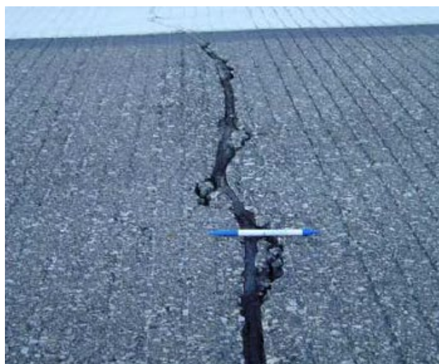
Figure 16. Longitudinal and Transverse Cracking
