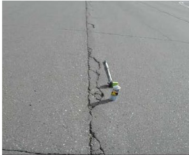
Figure 15. Joint Reflection Cracking from PCC
