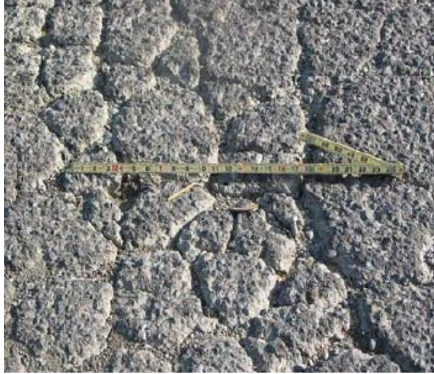
Figure 9. Alligator or Fatigue Cracking
