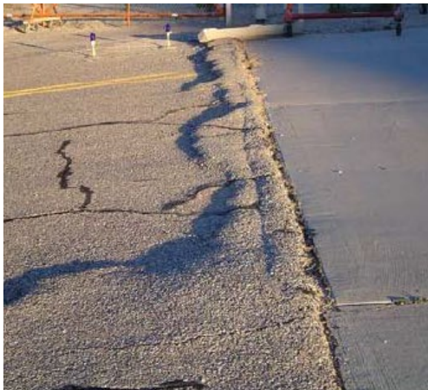
Figure 22. Shoving of Asphalt Pavement by PCC
