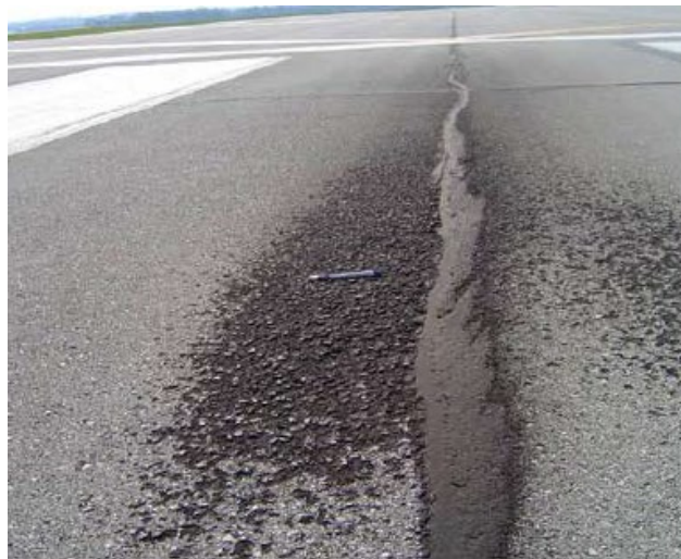
Figure 14. Jet Blast Erosion
