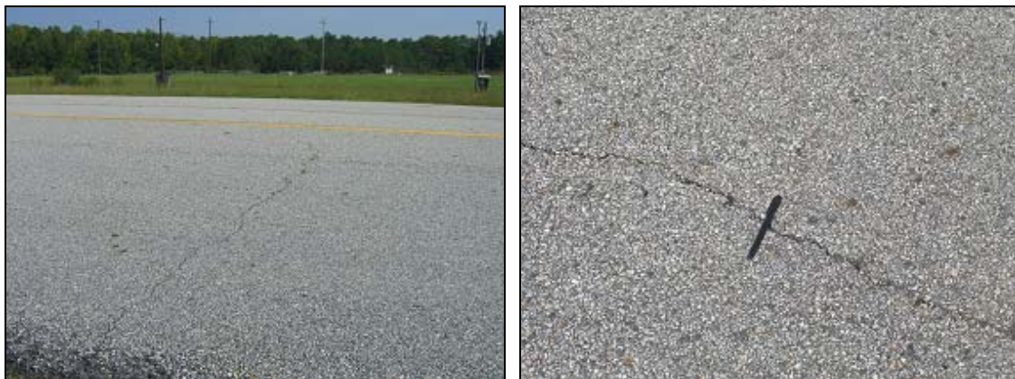
Figure B7 Transverse cracking along Taxiway A at Griffin-Spalding Airport
