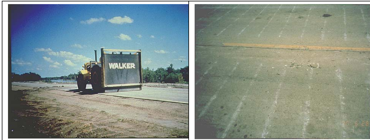
Figure 20. Crack and Seat or Break and Seat Equipment for Fracturing PCC Slabs
