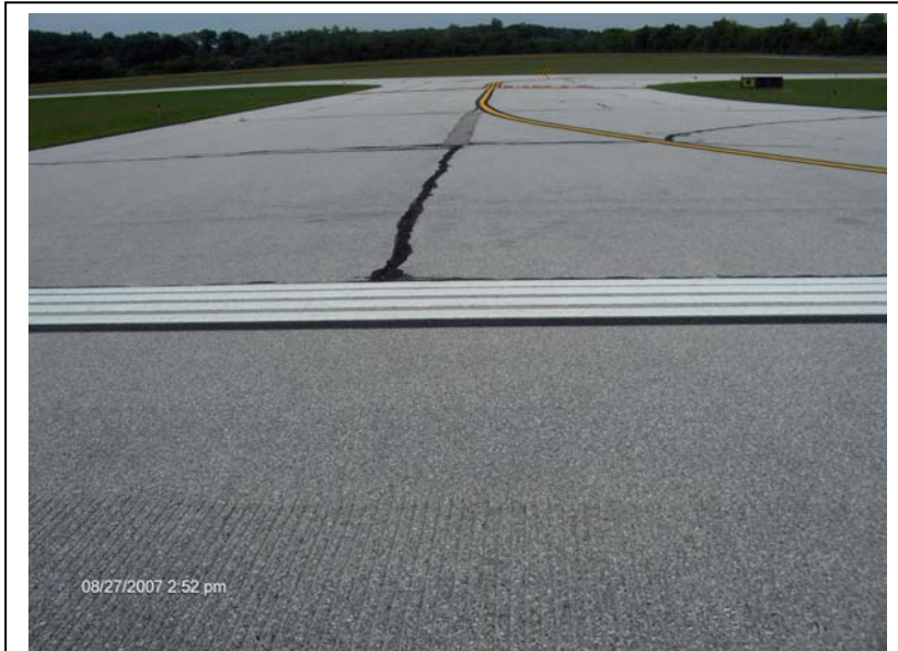
Purdue University Airport – PavePrep Section with 4-inch P-401 Overlay for Taxiway Rehabilitation.
