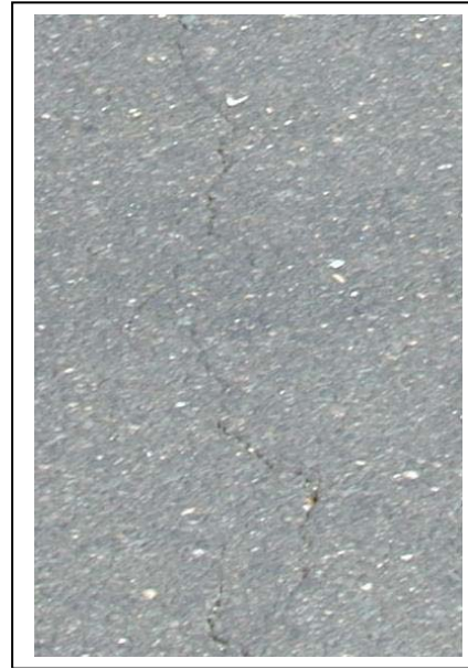
Hairline to Low Severity Reflective Crack—Crack can be seen and extends across paving width.
