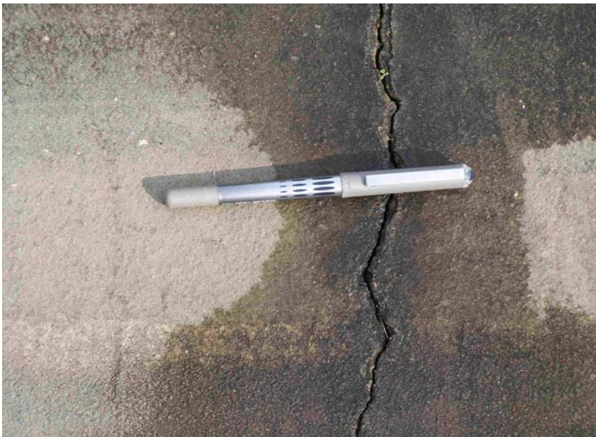
Figure 2-11 – Close-up of Block Crack Condition.
