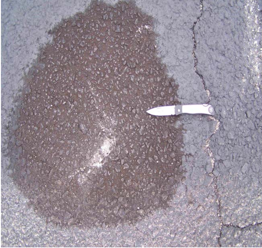
Figure 2-5 – Jet Fuel Stain on CarbonPlex Seal Coat, After Six Months.
