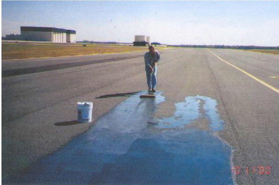
Figure 2-1– LAS-320 Application, TWM, McDill AFB, FL, 2003
