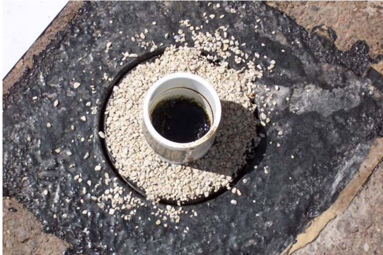
Figure 3-33 – Kitty Litter Used To Control Fuel Leakage
