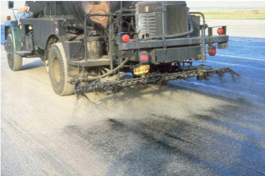
Figure 11.7 – Poor uneven application of tack coat
