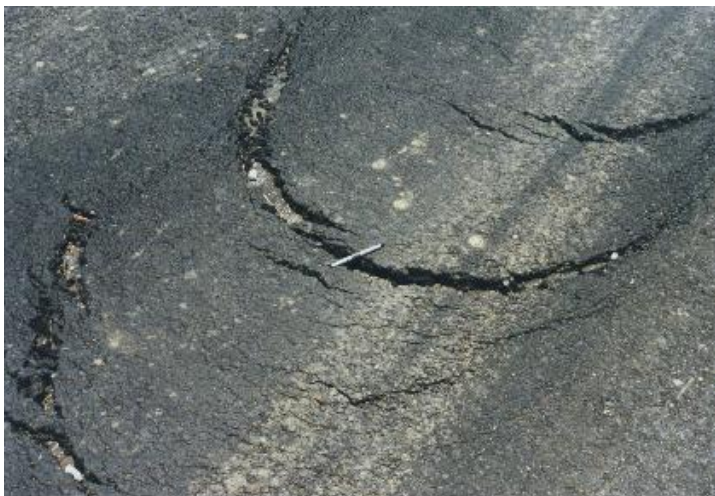
Figure 14.6 – Typical slippage problem
