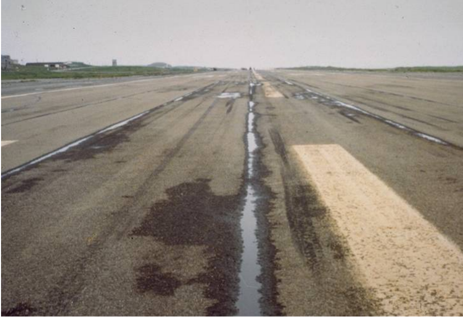
Figure 15.2 – Deterioration of longitudinal joint due to cracking and raveling
