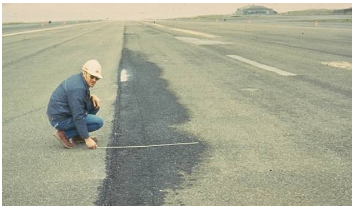
Figure 20.5 – Raveling next to longitudinal joint
