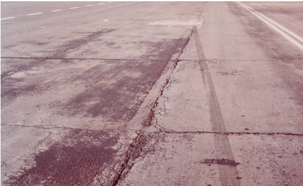
Figure 20.10 – Reflective cracks in HMA over existing concrete pavement
