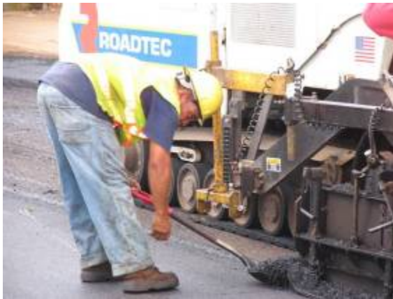
Figure 12.2 – Obtaining HMA in front of the screed on the side of the paver
