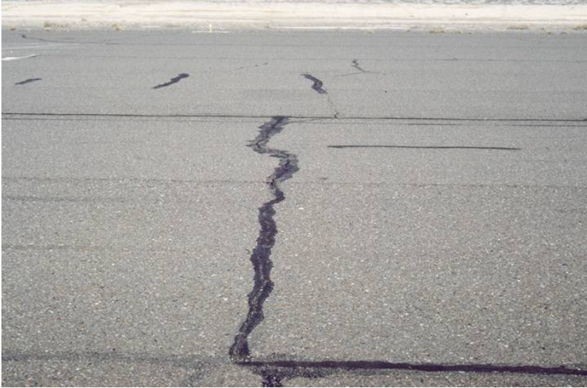
Figure 20.9 – Thermal cracking running in transverse direction
