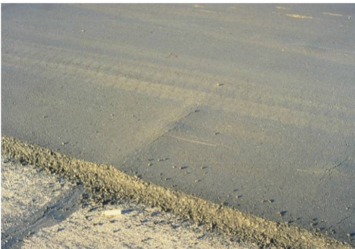
Figure 11.6 – Bump caused by excessive crack sealant
