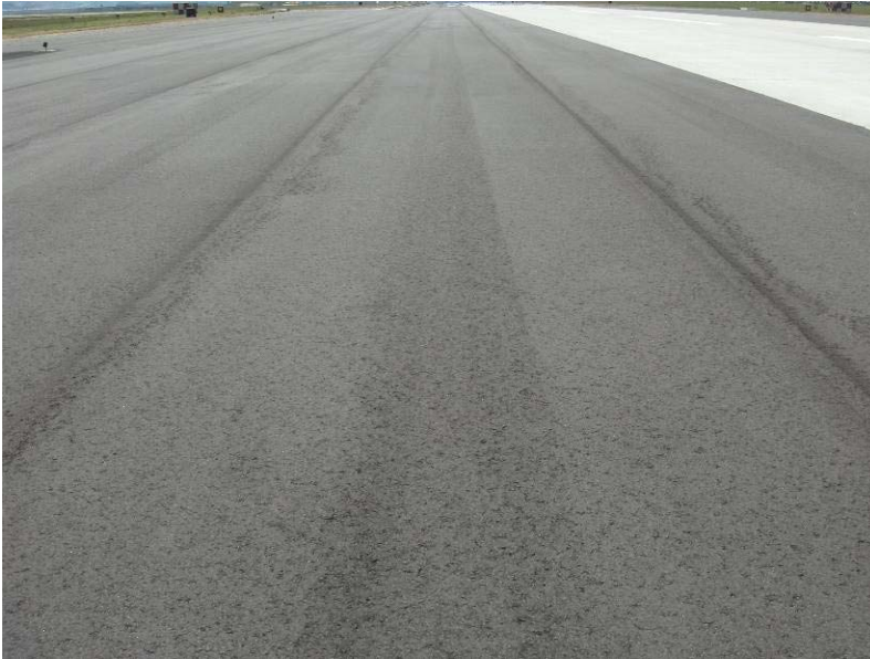
Figure 20.13 – Poorly constructed longitudinal joints
