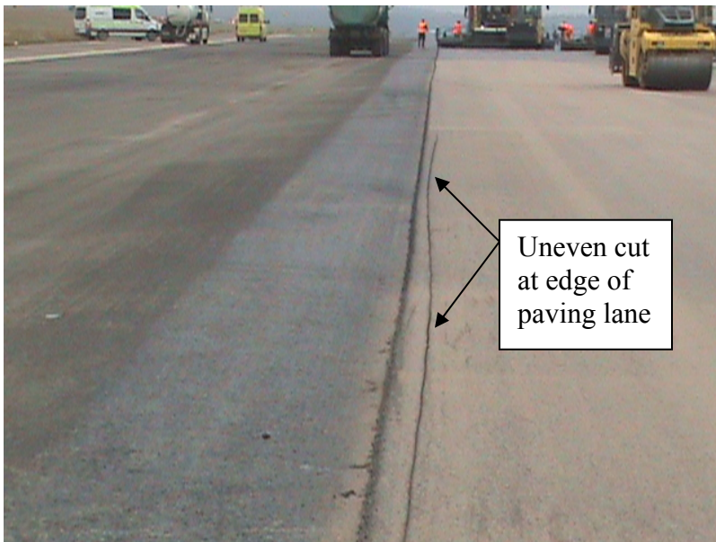
Figure 15.7 – Unacceptable cut of free edge
