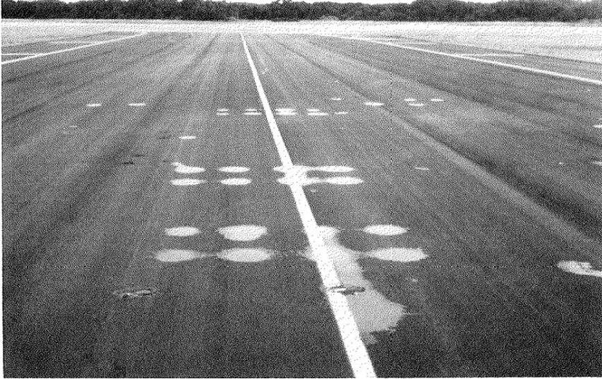
Figure 2.2 – Example of surface depressions caused by densification in the base course under a parked C-5 aircraft
