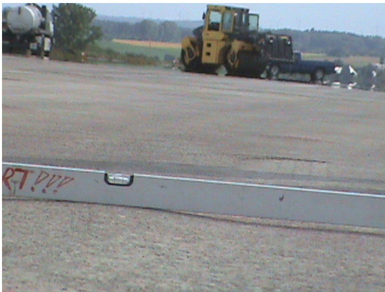
Figure 20.7 – Blister in newly constructed pavement
