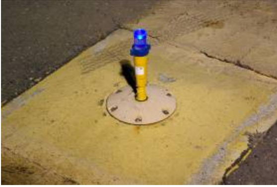
Figure 12.7 – Light fixture on a taxiway shoulder
