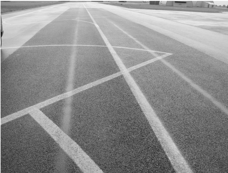
Figure 2.3 – Example of rutting caused by additional densification of an asphalt concrete by aircraft traffic (note water standing in ruts)
