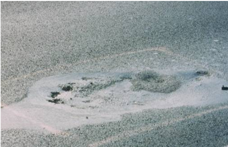
Figure 20.3 – Bleeding due to diesel contamination
