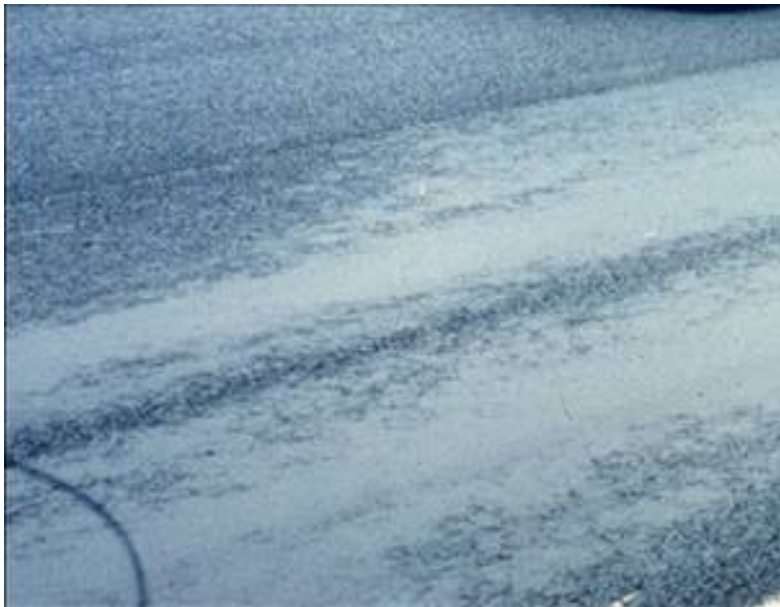
Figure 20.2 – Bleeding in an asphalt mixture
