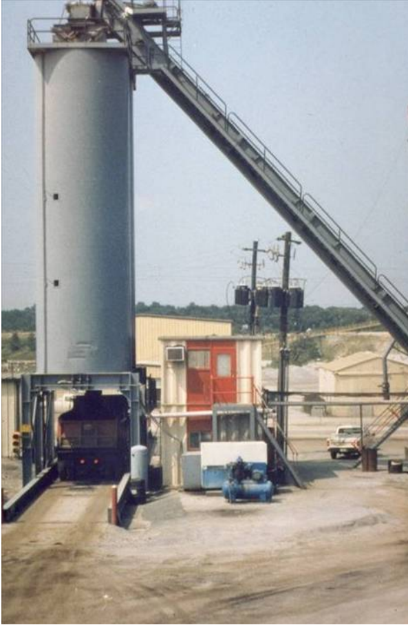
Figure 9.6 – Storage silo for HMA
