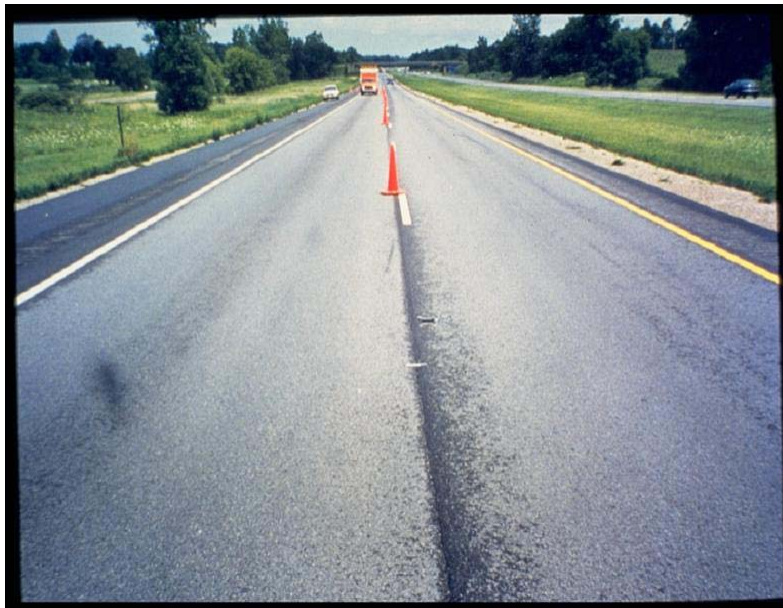
Figure 6. Raveling along longitudinal joint
