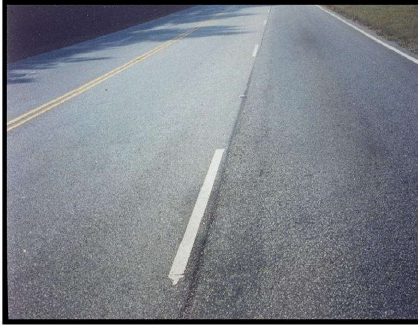
Figure 5. Raveling along longitudinal joint
