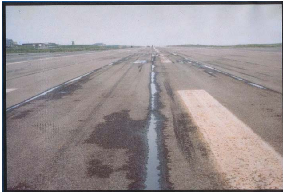
Figure 2. Deteriorated long joints on airfield runway
