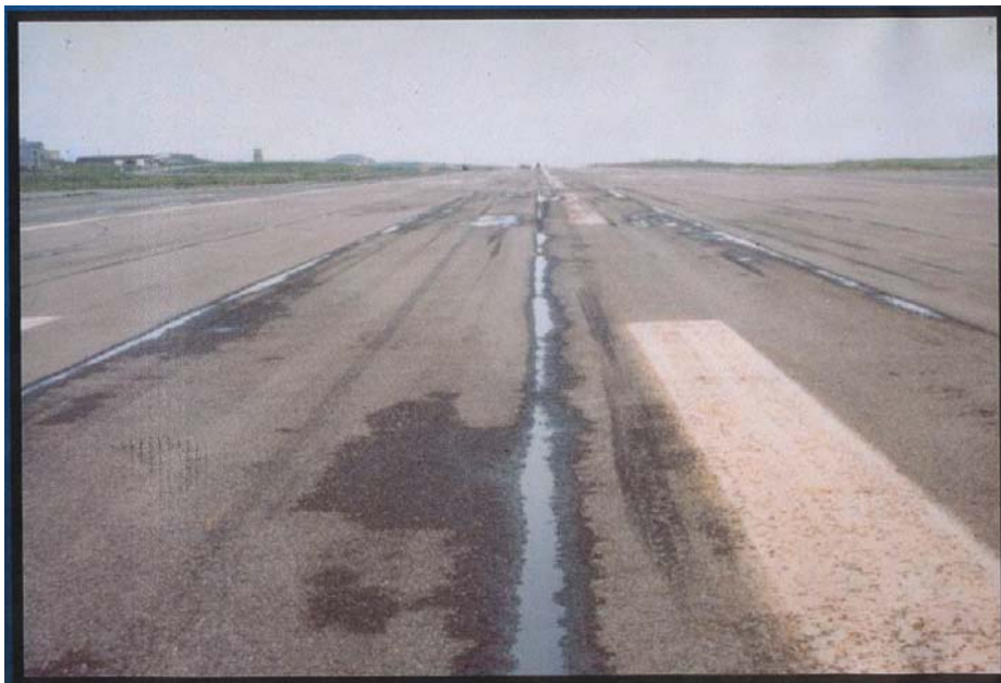
Figure 2. Deteriorated long joints on airfield runway
