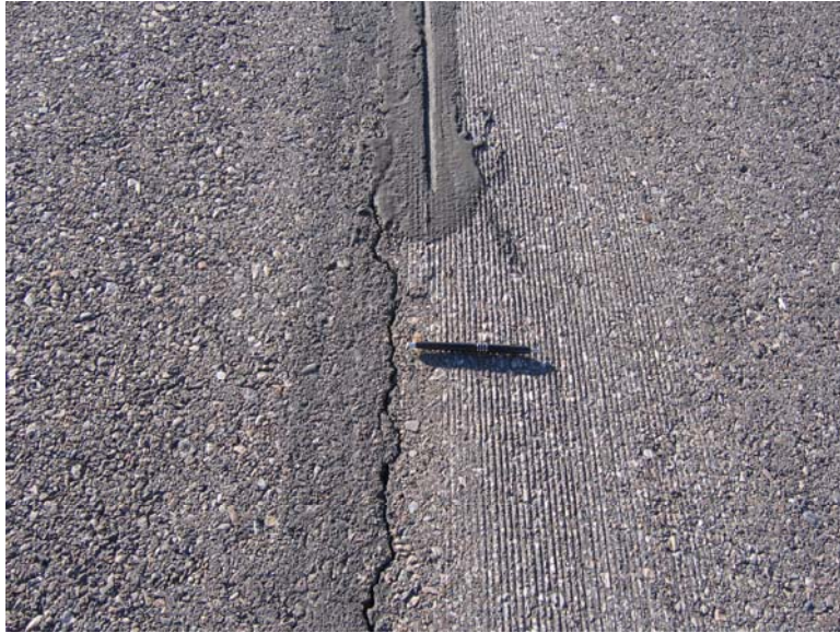
Figure 1. Low severity cracking in joints (Mt. Home AFB, Idaho)
