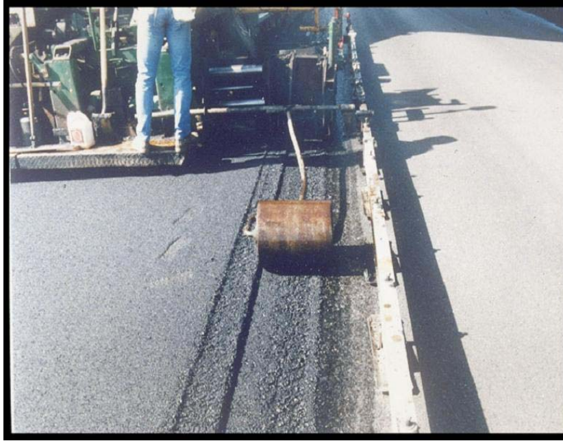
Figure 18. Small roller attached to paver compacts the taper of notched wedge joint
