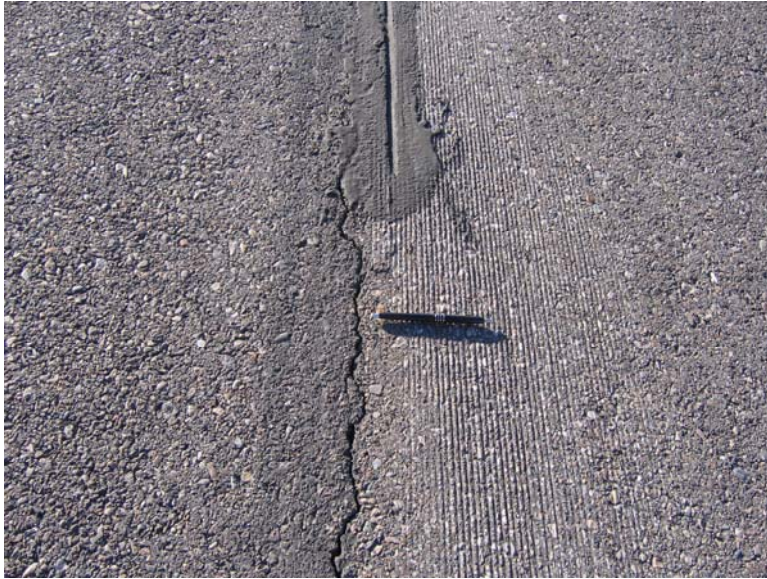
Figure 33. Low severity cracking in joints (Mt. Home AFB, Idaho)
