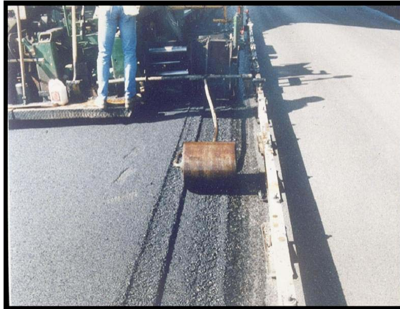
Figure 8. Small roller attached to paver compacts the taper of notched wedge joint
