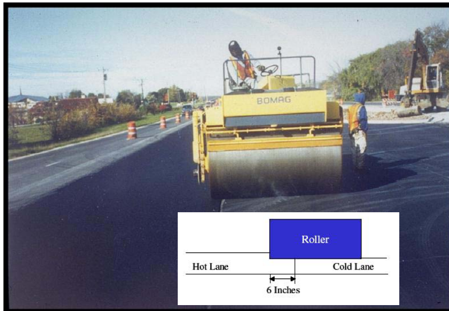
Figure 13. Rolling from the cold side with a 6-inch overlap on hot lane
