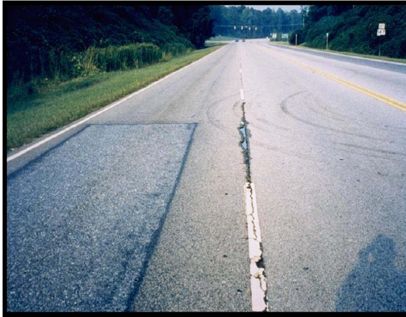
Figure 7. Intrusion of water through open longitudinal joint into the pavement system weakens its foundation requiring repairs
