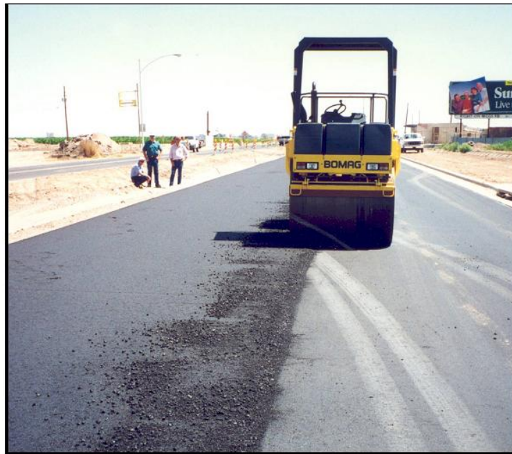
Figure 5. Bad practice of broadcasting the raked material onto the hot lane
