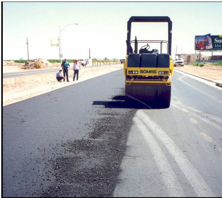
Figure 10. Bad practice of broadcasting the raked material onto the hot lane
