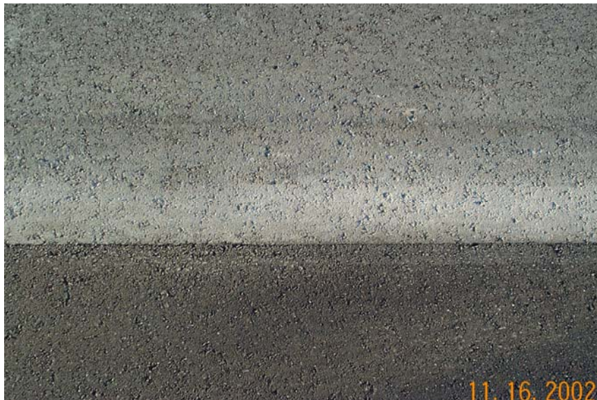
Figure 14. Improper joint with not enough material
