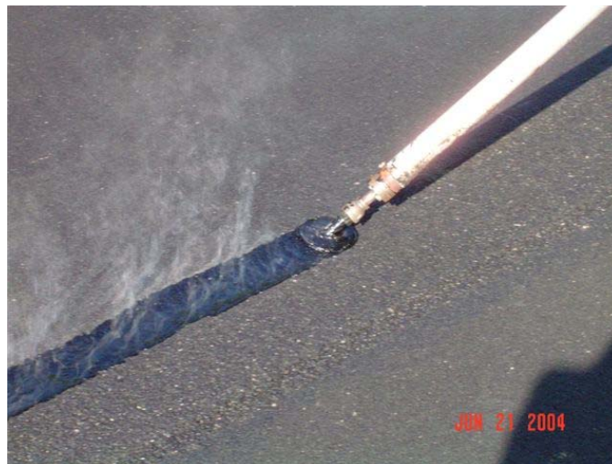
Figure 16. Close up of rubberized asphalt tack coat application on a notched wedge joint
