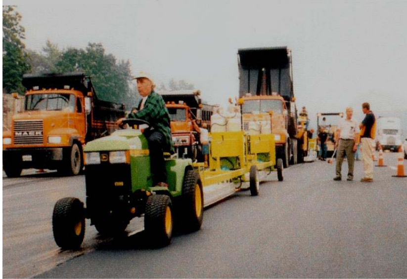
Figure 29. Infrared preheaters are towed with a small tractor ahead of the paver
